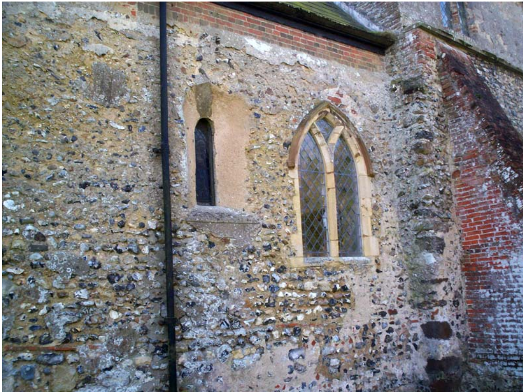
Plate 2. The north wall of the chancel showing the double splayed lancet window, the blocked circular window to the left, the course of Roman brick below and the north-east corner of the nave
