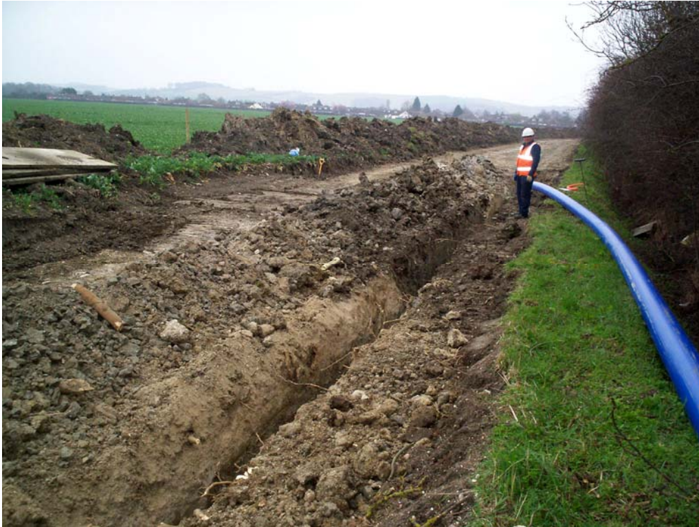
Plate 3. The water main being laid in the area of the gas main, looking south
