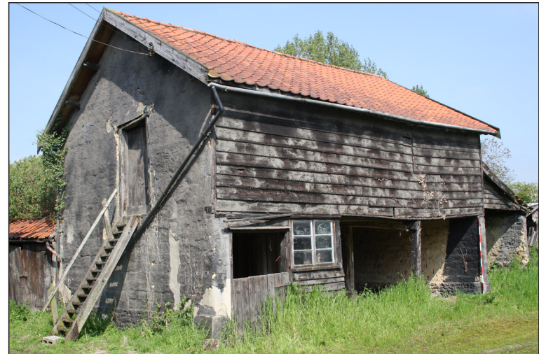
Plate 12. Front elevation of the barn showing the two storey hay loft and cart store. Facing north-west
