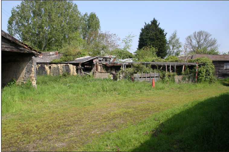
Plate 9. Degraded outbuilding. Facing north-west.
