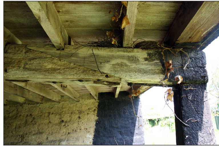
Plate 30 a. The principal beam shows evidence of failing at some of these old tenon joints.
