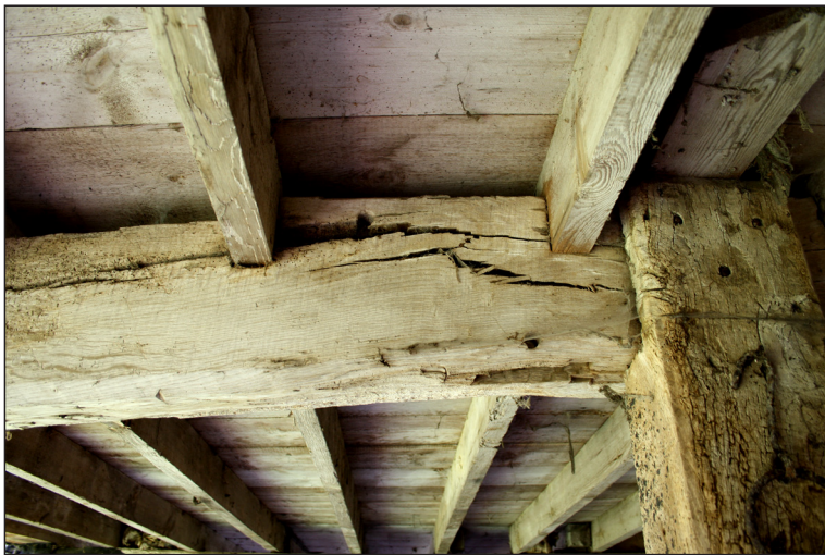
Plate 30 b. There is evidence of previous repair with a large scarf joint above the front post.
