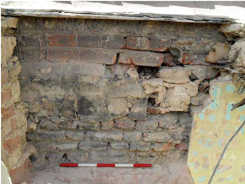
Plate 9. Detail of wall following removal of render at north end of east cloister wall, looking west, 0.50m scale
