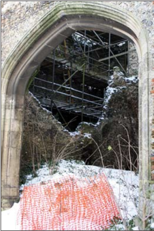
Plate 13. Pre-excitation view showing collapsed internal west wall
