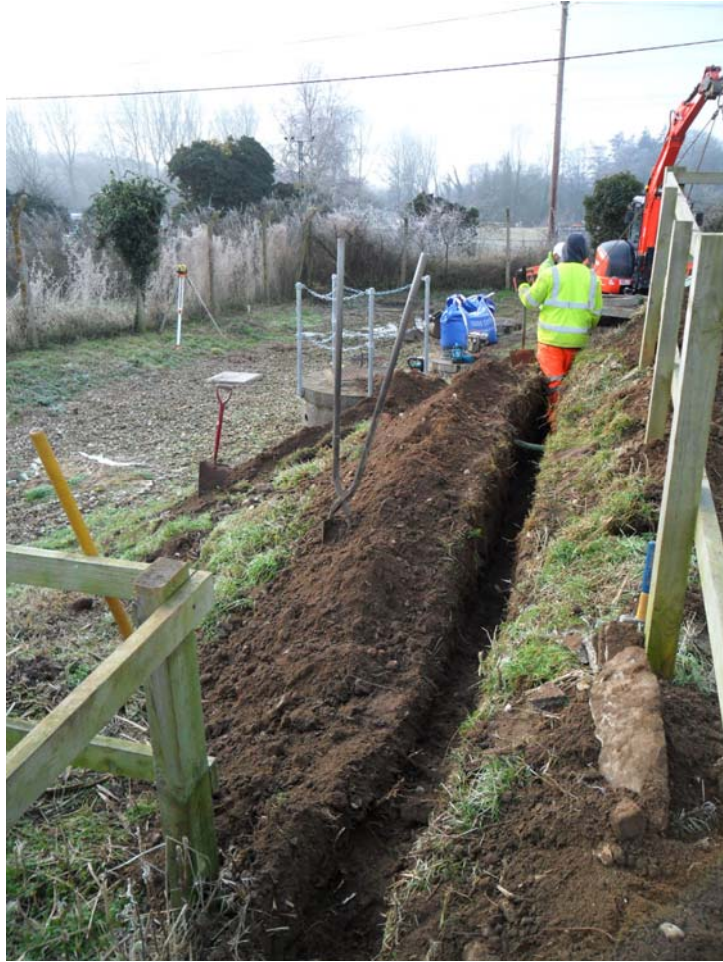
Plate 2. The service trench running across the southern slope of the mound, facing west
