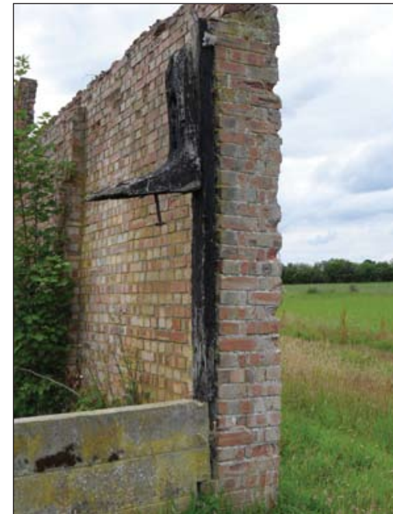
P8. Close-up of possible re-used timber in modern rebuild of east wing B, looking west
