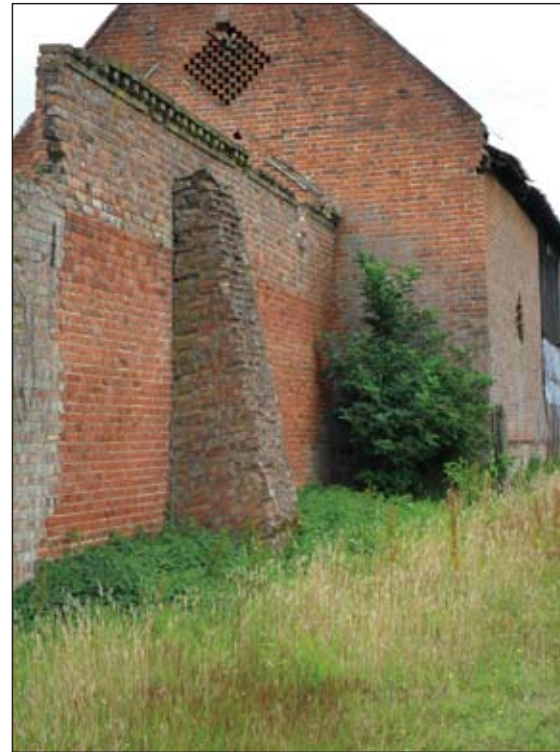
P10. Side wing and main barn, showing modern buttress and rebuilding to wing, looking south
