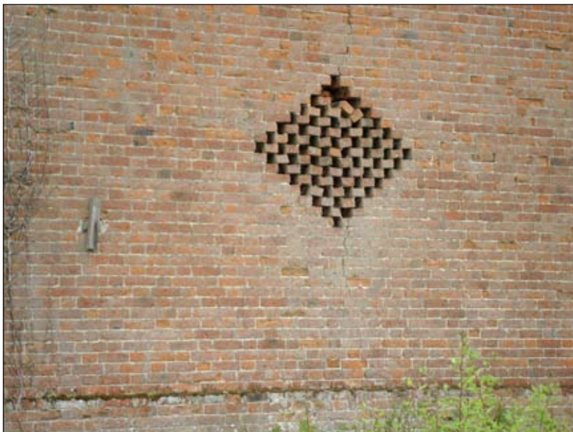
P15. Close-up on right hand un-blocked ventilation hole on north-western elevation of main barn, looking south-east
