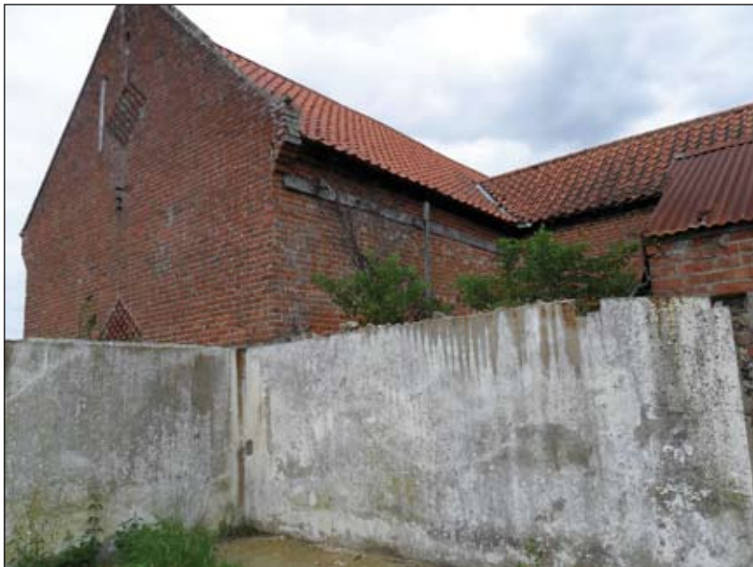
P19. Inside western yard, looking up at western gable of main barn and western lean-to, looking north
