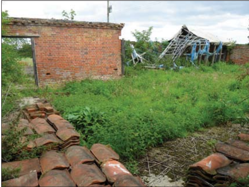
P32. South-eastern yard shoring part of east wing B and the shell of east wing A, looking east
