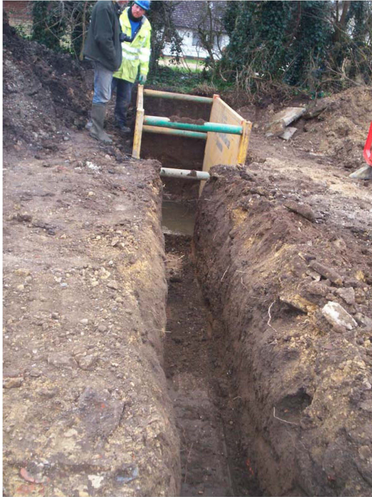
Plate 5. The open-cut trench and the final joint bay facing south, with pit [30] visible in the base of the trench
