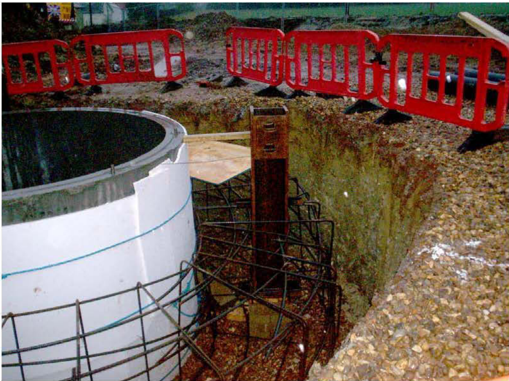
Plate 2. The installed wet well
