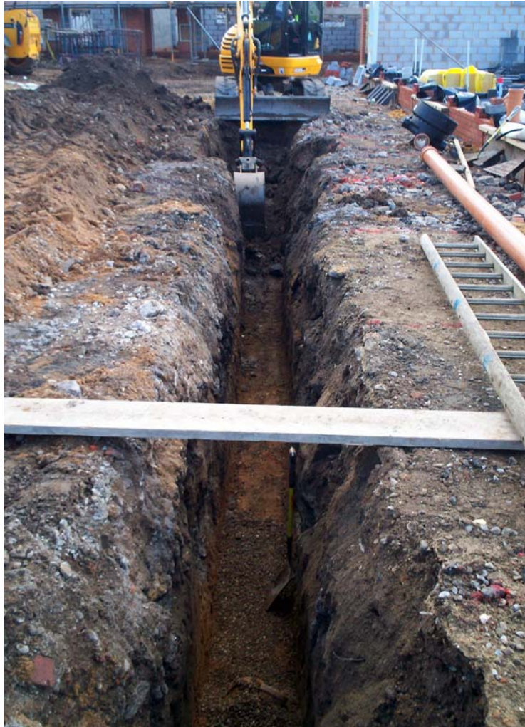
Plate 1. The sewage trench facing east (the machine bucket is at the western end of the cellar)
