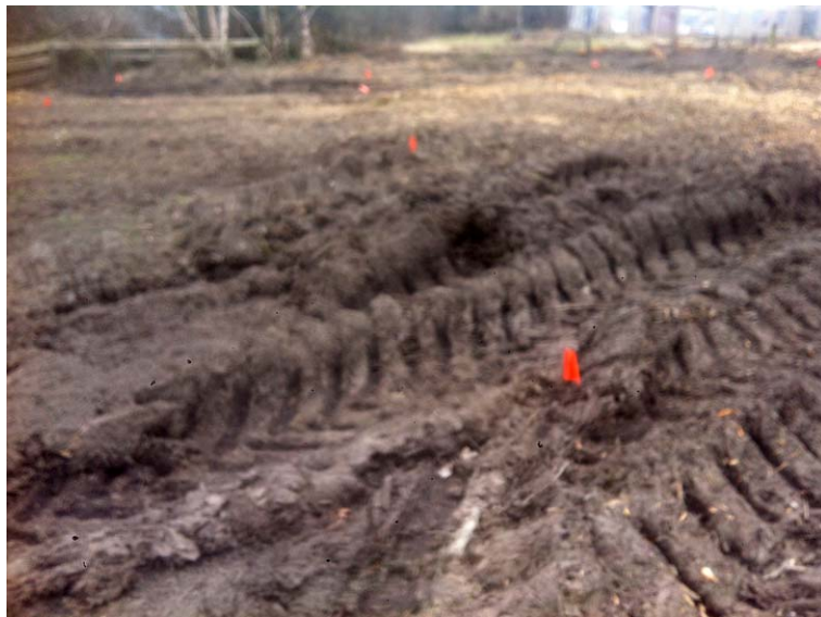
Plate 4. Soils churned up by heavy plant
