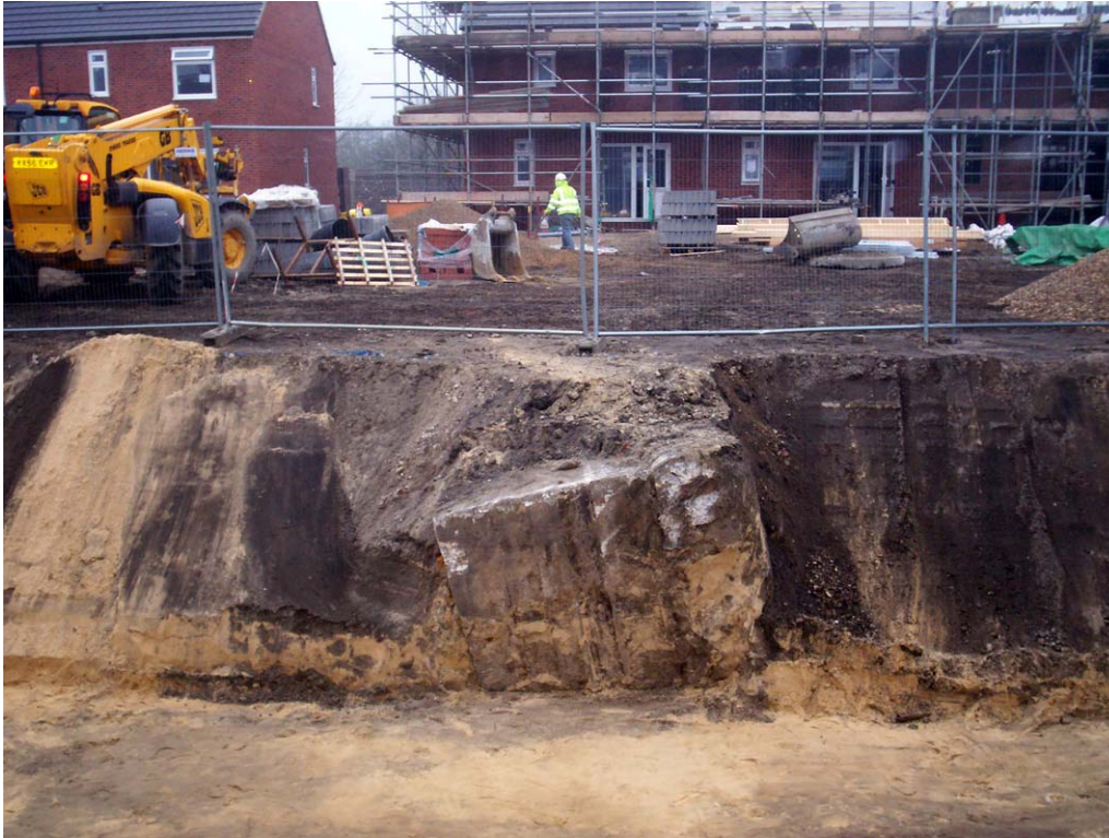
Plate 5. Soakaway with the displaced concrete block, facing west
