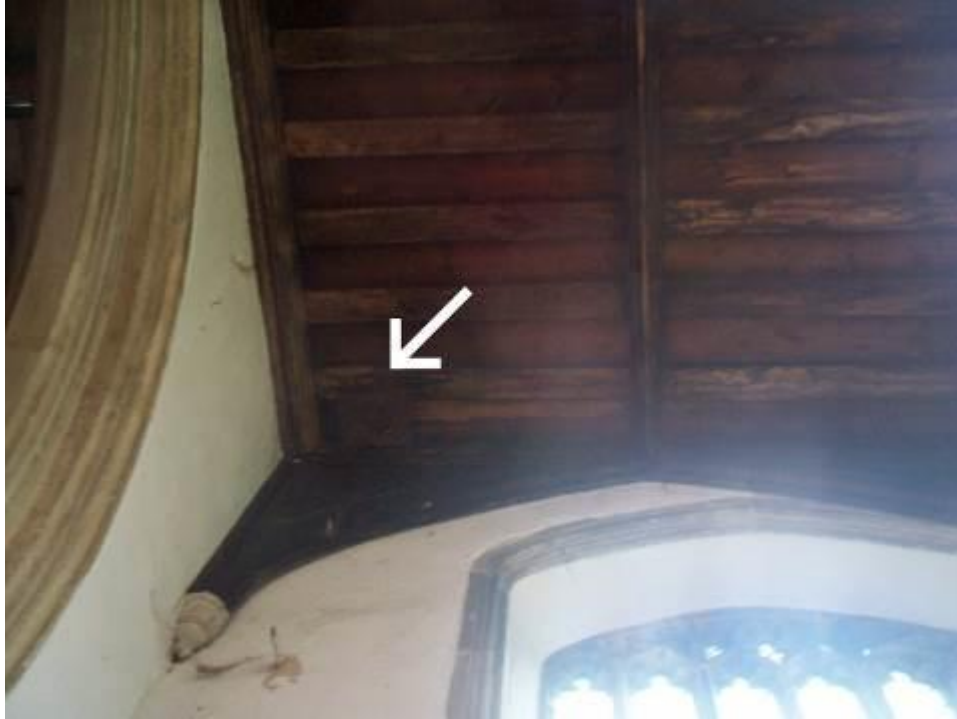
Plate 4. Hole in the medieval roof (arrowed), perhaps for a stove flue
