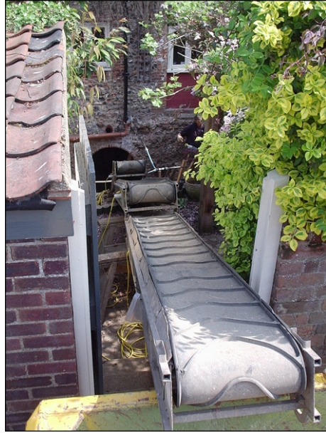
Plate 1 End of conveyor belt at rear of property
