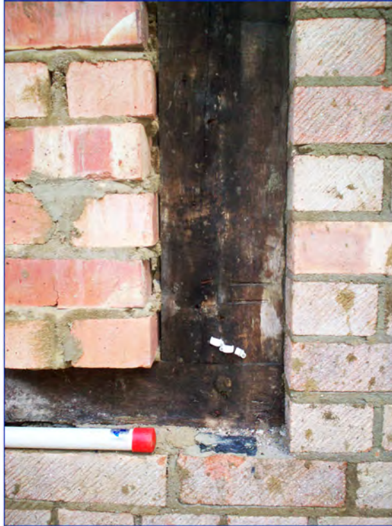
Plate 13 Detail of timber framing, showing mortice-and-tenon joint with peg and carpenter's assembly mark
