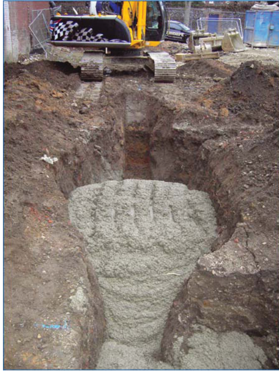
Plate 1 Foundation trench widened due to collapsed edges
