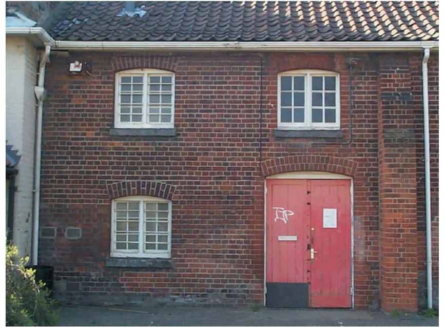
Plate 7 First two bays at south-west end of Malthouse showing renewed door and window and later buttresses
