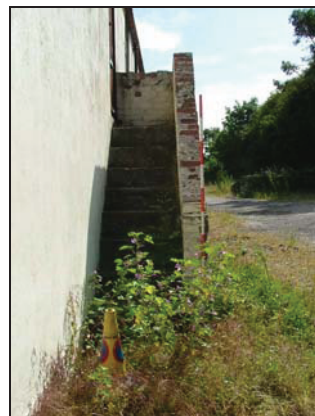
Plate 12. Concrete steps set in a brick surround, south elevation of Building B
