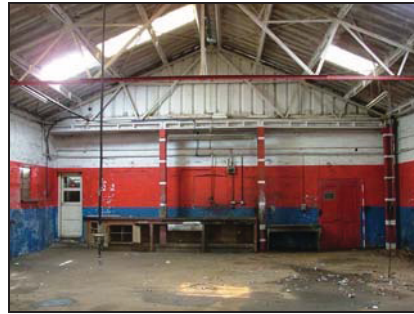
Plate 40. North wall of Building B as seen from the interior of Building D
