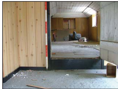
Plate 42. Difference in floor level between Buildings A and B
