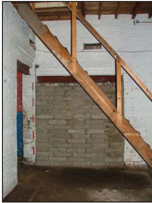
Plate 29. View west showing stairs to 1st floor at north end of Building A
