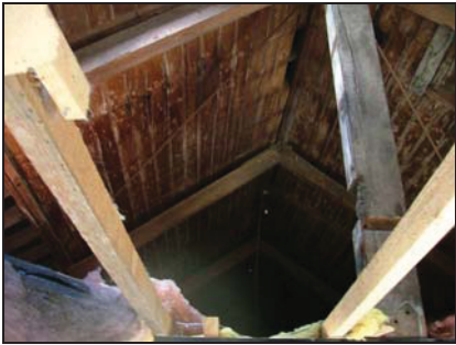
Plate 39. Detail of roof structure as seen from the south end of Building A
