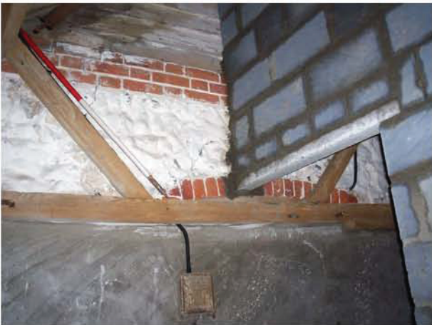
Plate 9. Dividing wall showing top of arch between Building B and C, 1m scale
