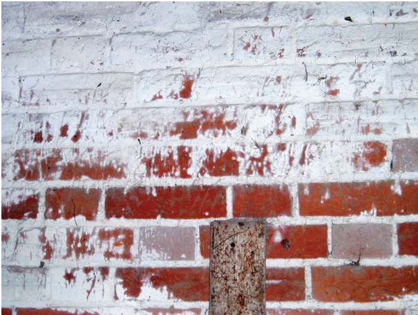
Plate 1. Vertical scratches on exterior west wall of Building A
