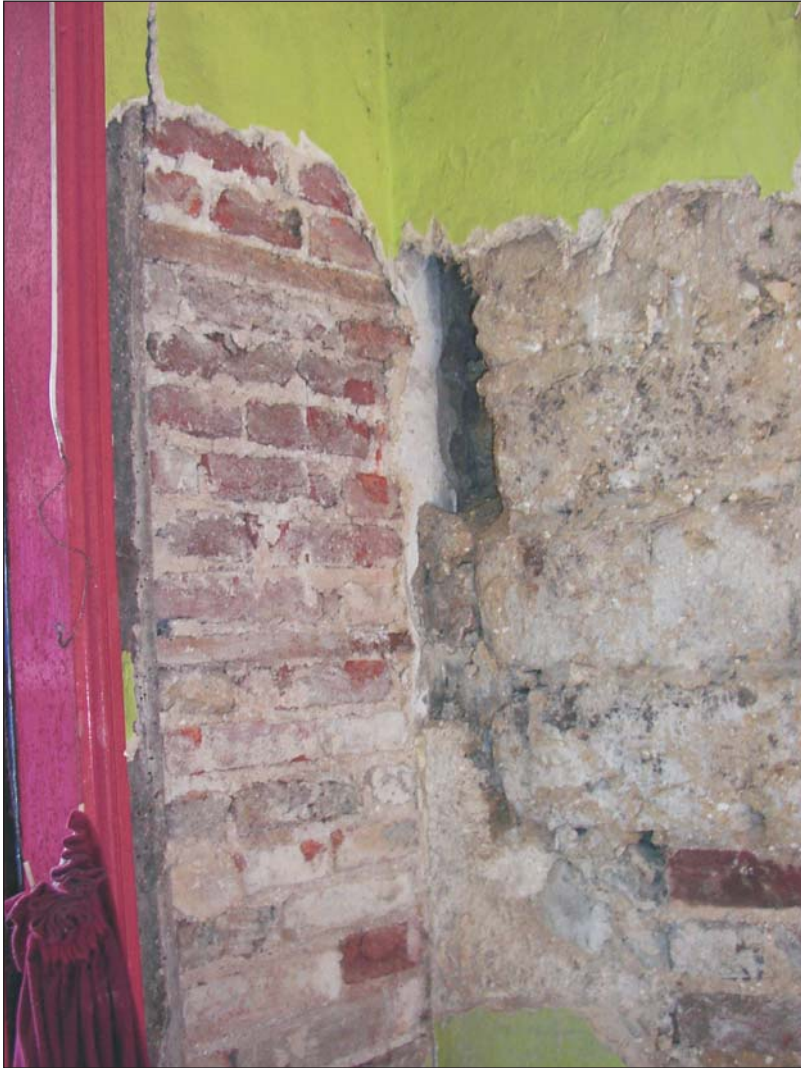
Plate 11. Junction of the brick wall of the south service room and the south wall showing the apparent anomaly of the plastered surface extending beyond the face of the outside wall
