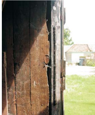
Plate 19 Building F3 looking south through doorway in south wall, showing in situ rollers
