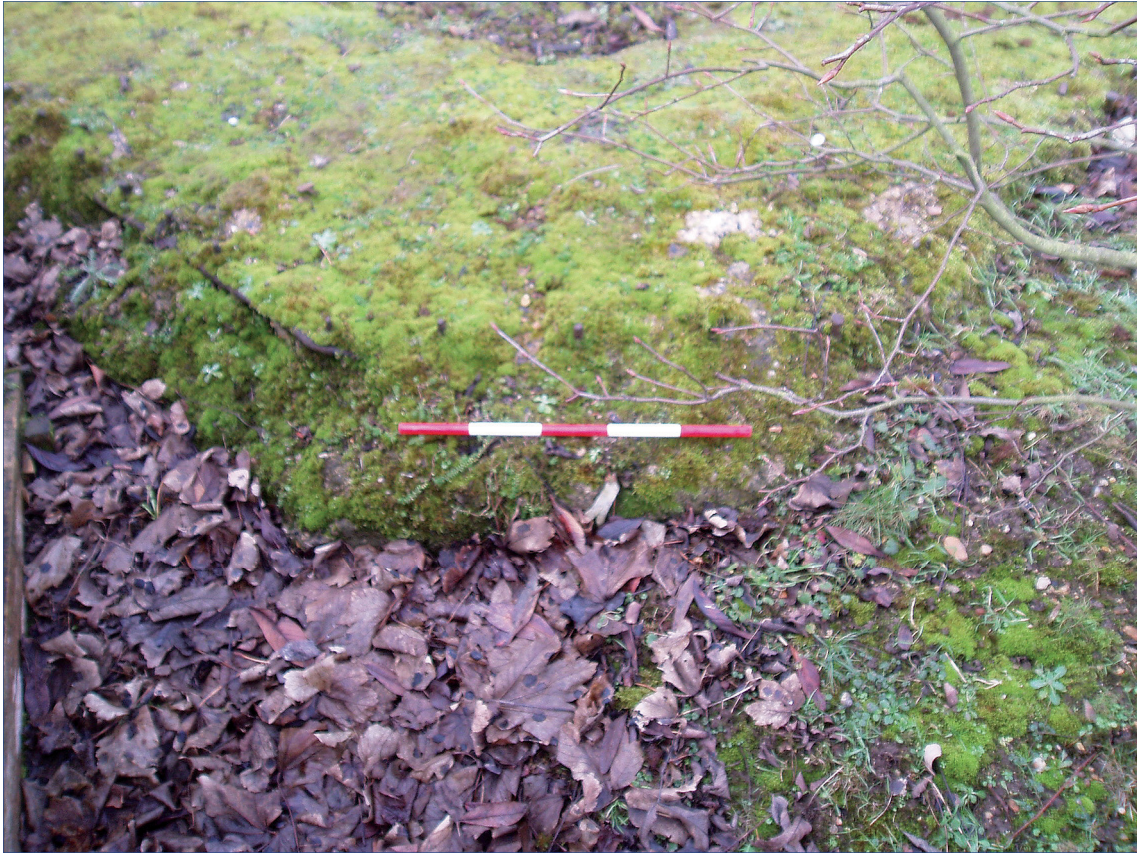
Plate 7 Looking west at the east corner of the pillbox base with reinforcement showing
