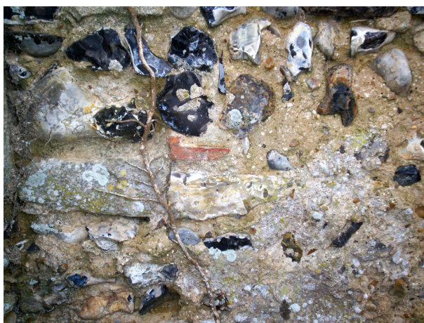
Plate 3. Chancel wall of the parish church showing reused Roman masonry and undated limestone blocks
