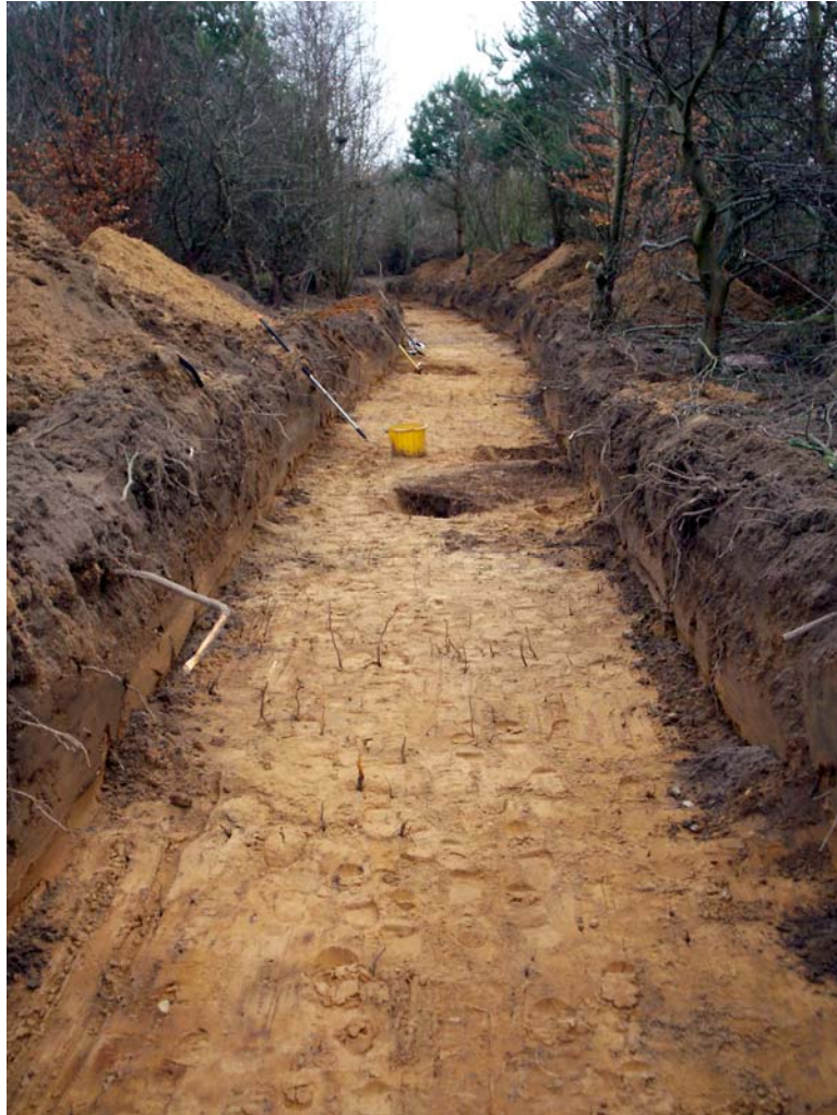
Plate 13. Looking south-east along the 2m wide easement through the wooded area adjacent to the electricity substation.
