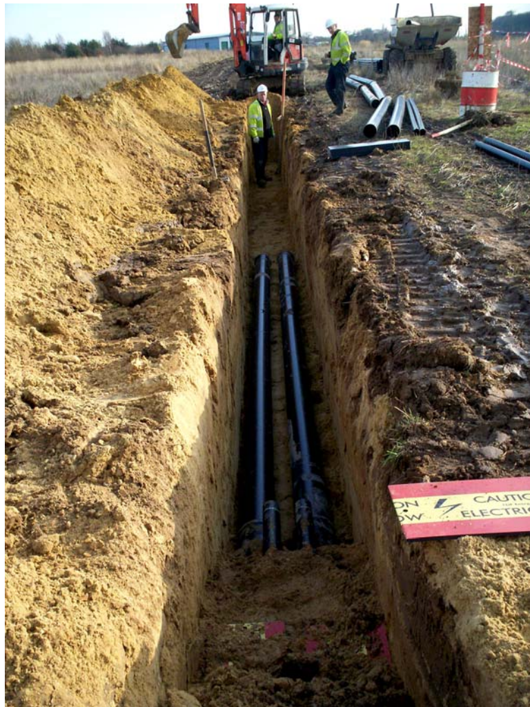
Plate 1. View of the trench with cable ducts, looking south-east towards the ambulance station.
