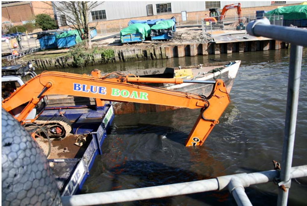
Plate 4. Excavation of trench across river bed, looking north from south bank of River Wensum
