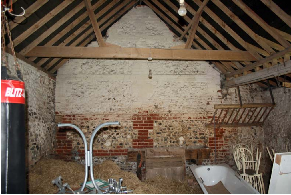
Plate 5. Eastern wall of western cell Building B1 showing hay rack and trough
