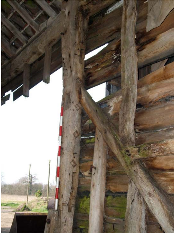
Plate 5. Post with mullion sockets east of cart door, looking north-west. 1m scale
