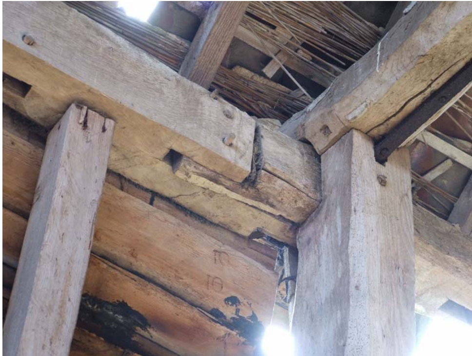
Plate 7. Face-halved and bridled scarf joint in south-east wallplate
