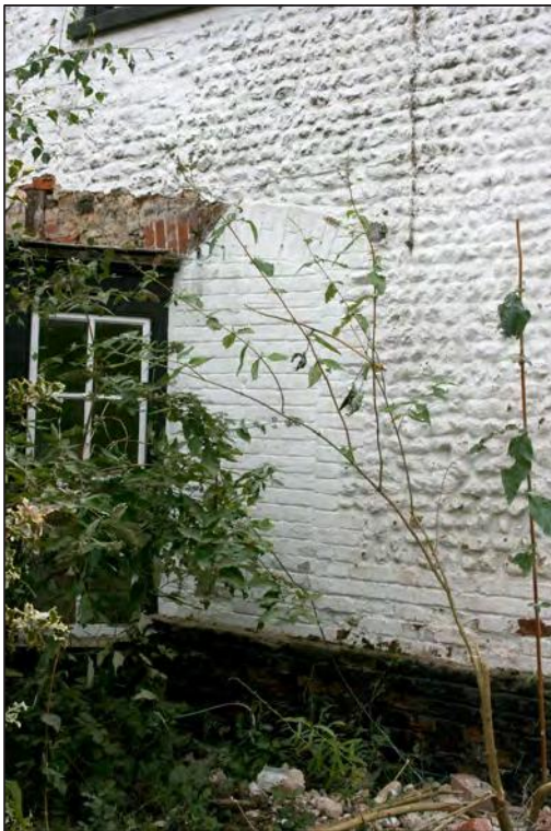
Plate 7. Blocked window beside bay window
