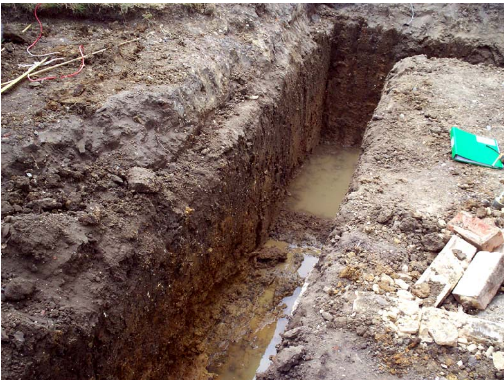
Plate 3. Trench at the south of the building where the base was particularly wet
