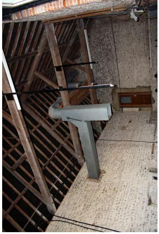
Plate 72. Building A extraction duct
