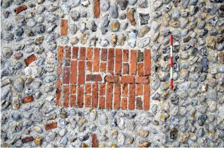
Plate 114. Blocked vent on Building A, 0.5m scale
