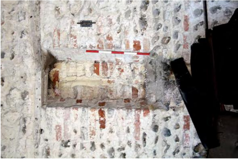
Plate 73. Building A blocked vent, 0.5m scale
