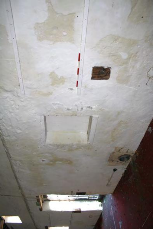
Plate 89. Building B blocked window, 0.5m scale
