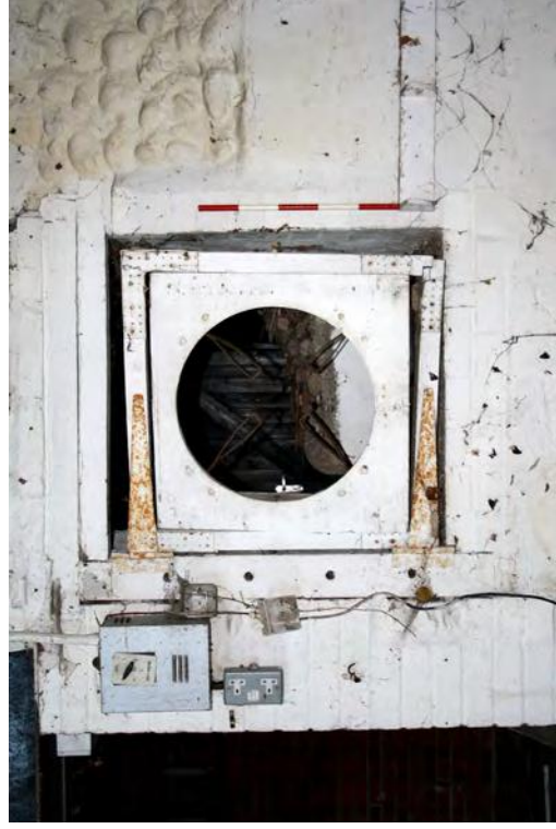
Plate 59. Building A Interior extraction fan facing east, 1x0.5m scale
