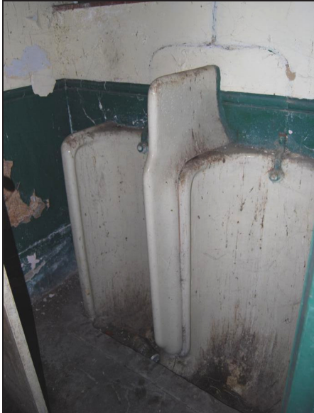
Plate 11: Original Toilet Furniture.
