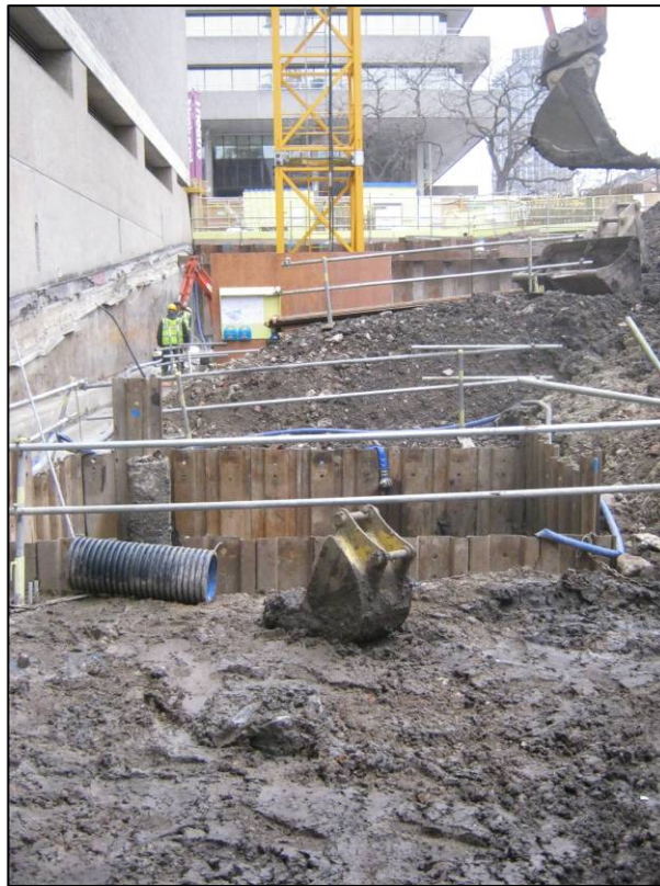
Plate 1: The formation level for the new basement, looking east, showing the scar of the access ramp on the existing rear wall of the theatre
