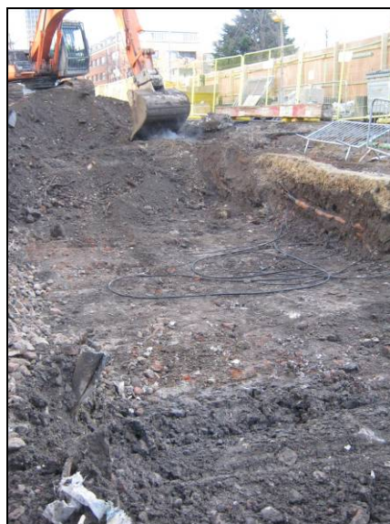
Plate 4: Ground reduction through modern made ground to the south of the basement, looking south-east
