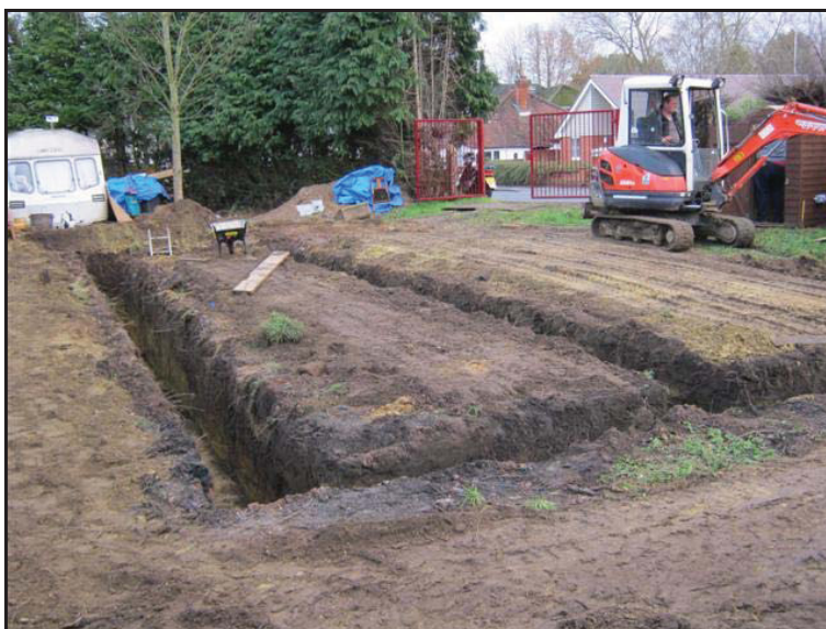
Plate 1: General view of excavation area from north-west corner of site (direction south-east)
