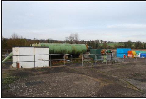
Plate A. General Shot of Tanks Looking West
