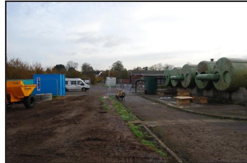
Plate B. General Shot of Tanks Looking South
