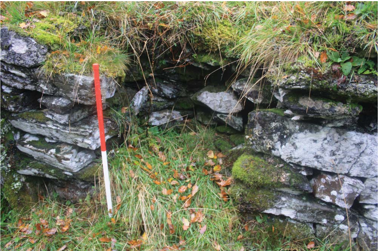
Plate 4: Detail of the collapsed cell in the SE-facing elevation, S entrance
