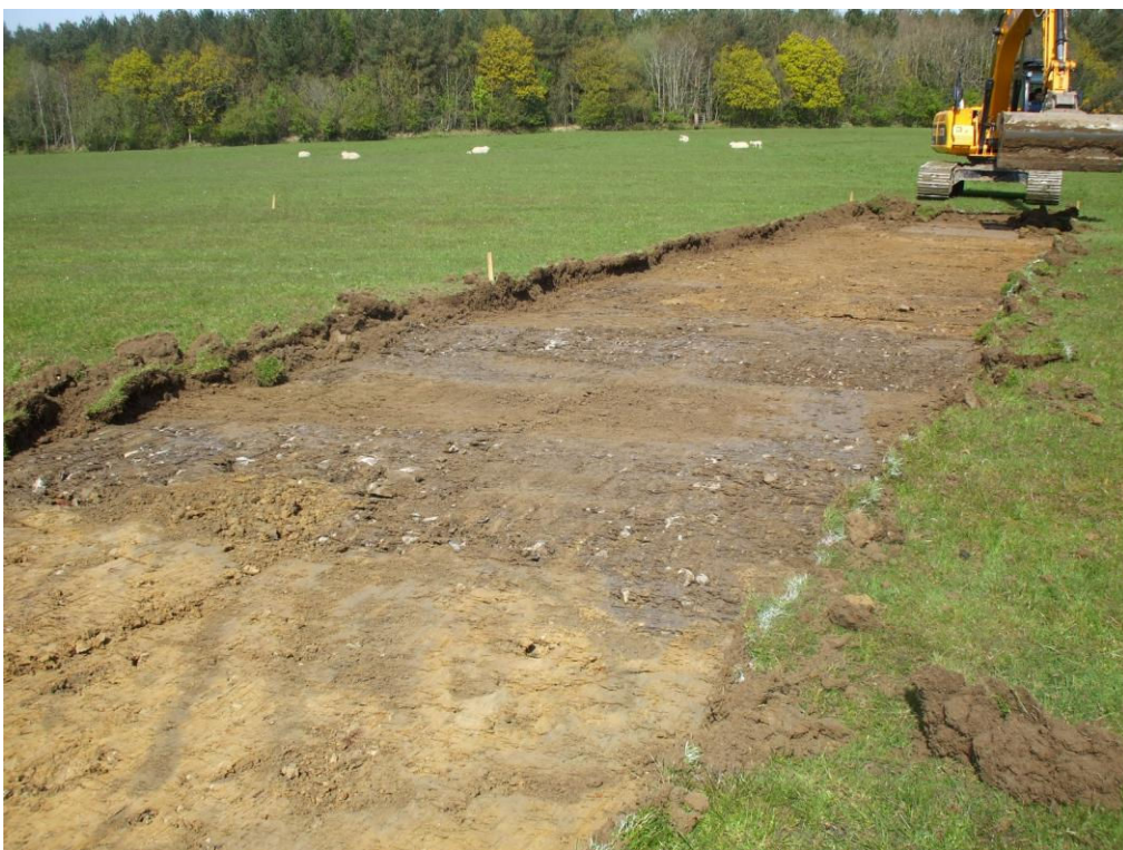
Plate 3 - Sewer cut within haul road 2
