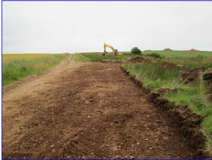
Plate 1: General view of strip of the initial haul road, from the north
