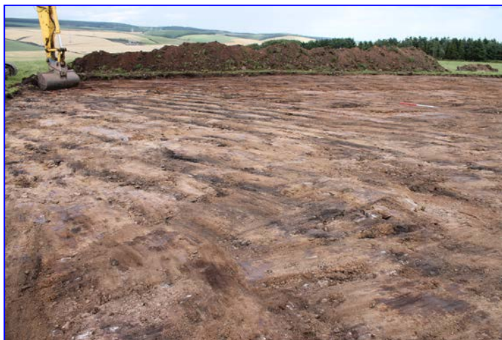
Plate 2: General view of completed strip of WGT3, general view of completed strip from the south-west, showing the deep plough marks
