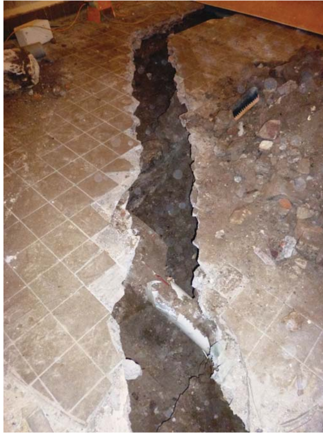
Plate 13: Cannonball House, lower ground floor, detail of the service trench exposing Wall [003] from the south - note that a modern brick and concrete service is located below this to the south
