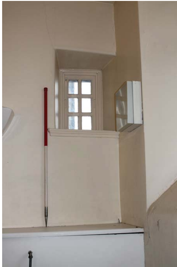
Plate 7: Cannonball House, detail of small early window to toilet block to the south in the south side of the east wall, from the west
