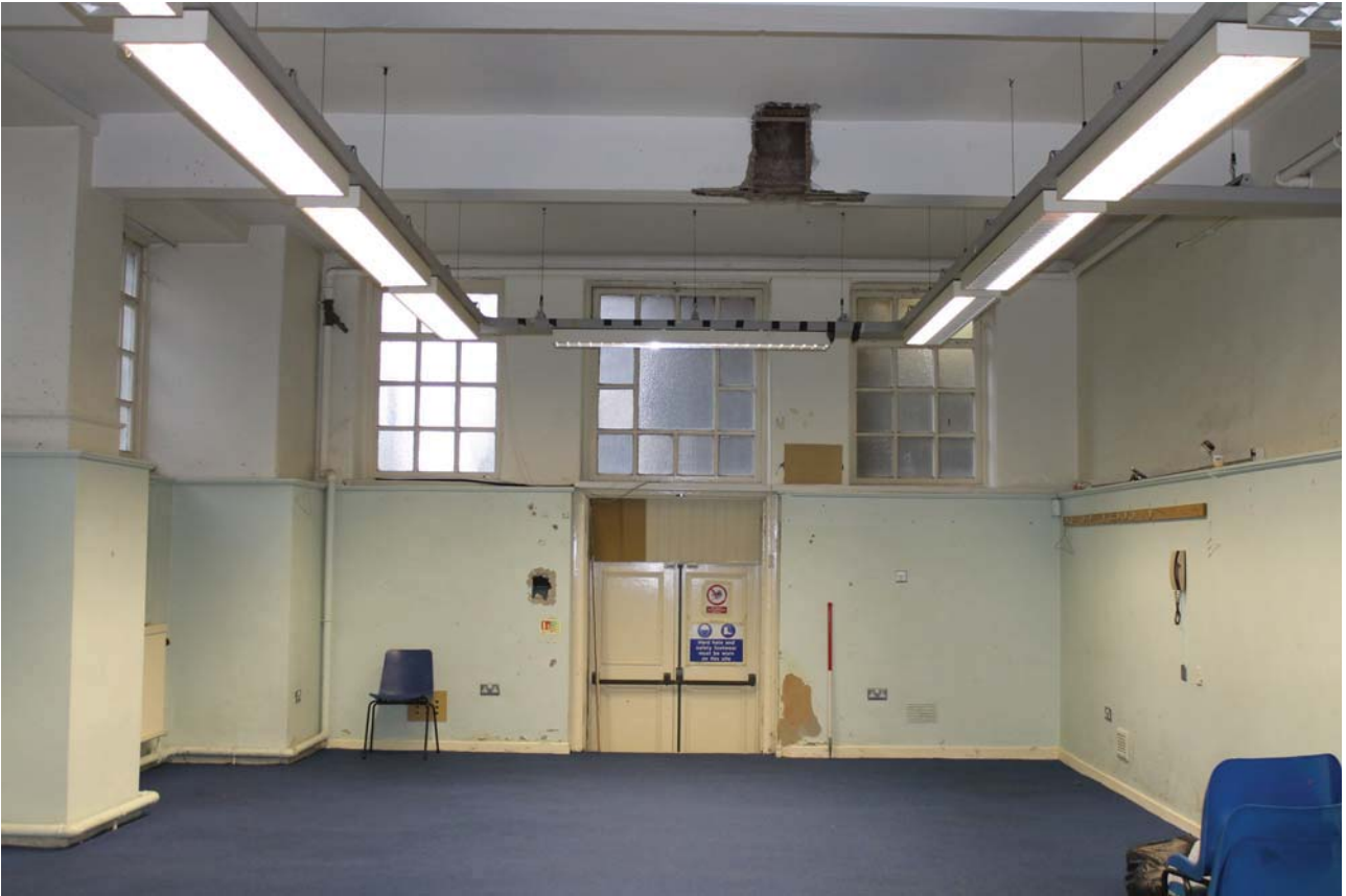
Plate 1: Cannonball House, lower ground floor, general view of the westernmost room from the south
