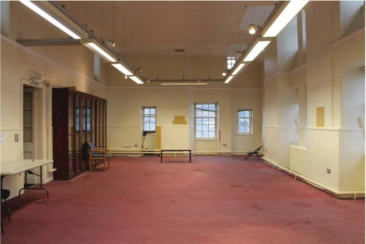
Plate 9: Cannonball House, first floor, general view of the westernmost room from the north
