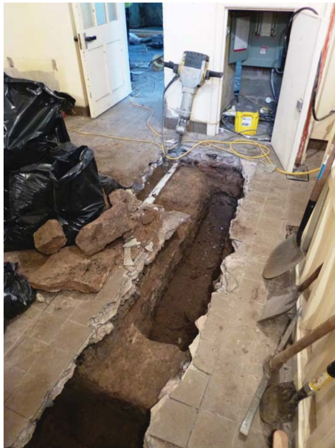
Plate 12: Cannonball House, lower ground floor, detail of the service trench exposing Wall [001] (to the foreground) and Wall [002] (running perpendicular to it from Wall [001], from the south)
