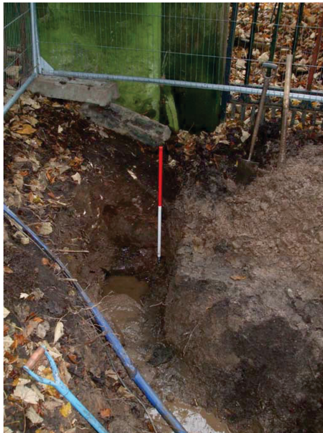
Plate 10: Detail of exposed stone culvert [026] adjacent to the east gate from the west
