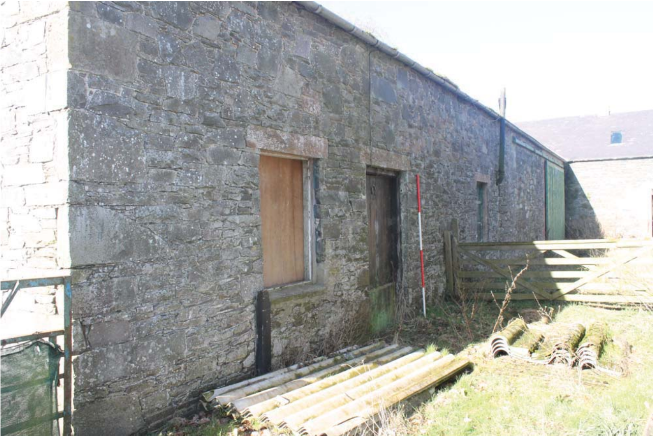
Plate 47: Barn C, east elevation, general view to the south side, from the south-east
