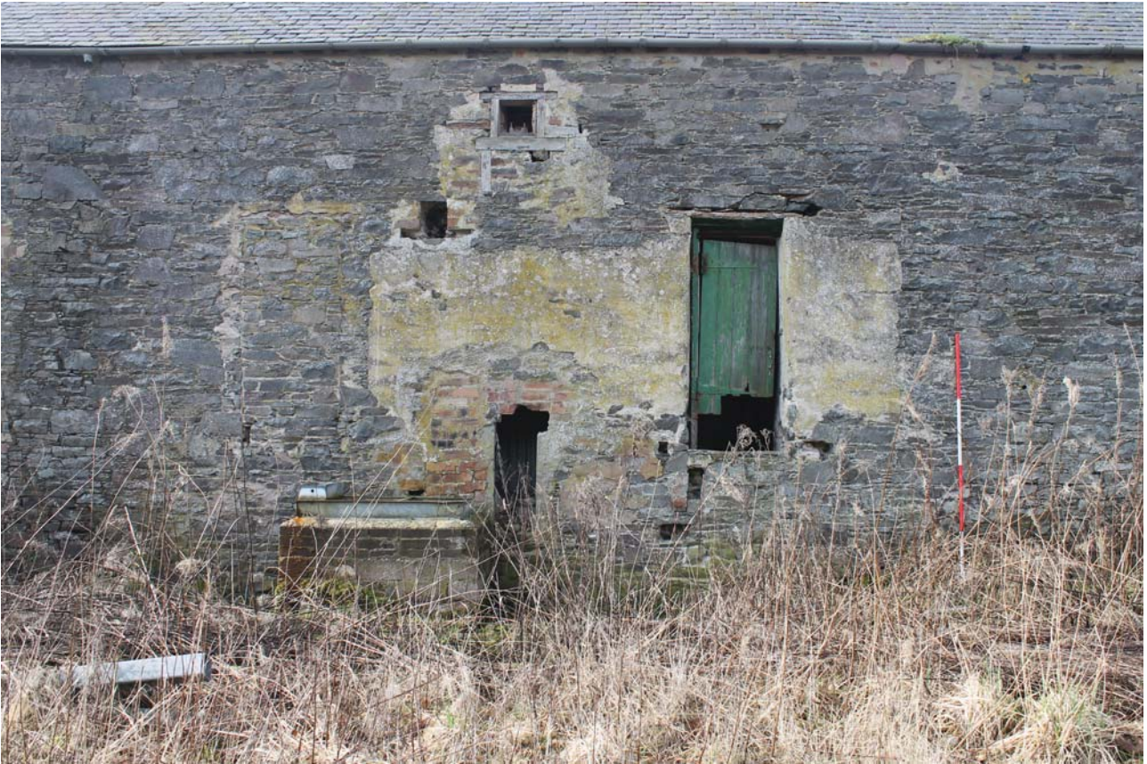
Plate 5: Barn A1, east elevation, detail of the openings and features associated with the water wheel from the east
