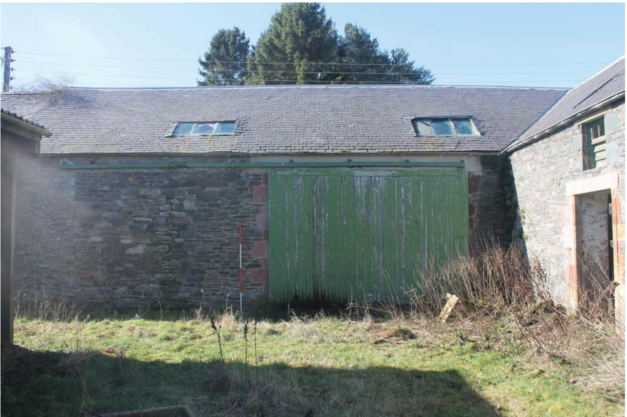
Plate 46: Barn C, east elevation, general view to the north side, from the east
