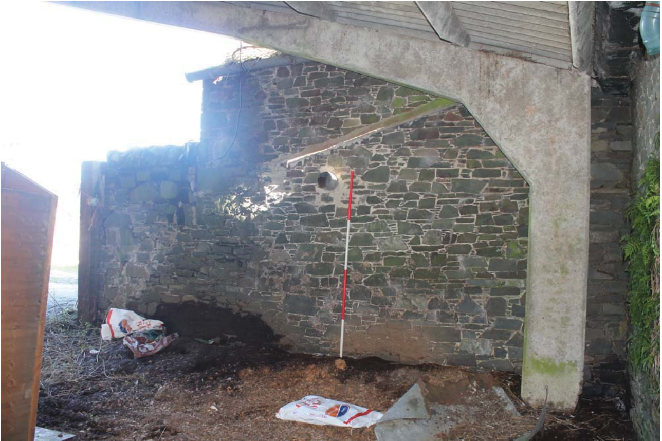
Plate 11: Barn A1, west elevation to the north side, general view from the SWW
