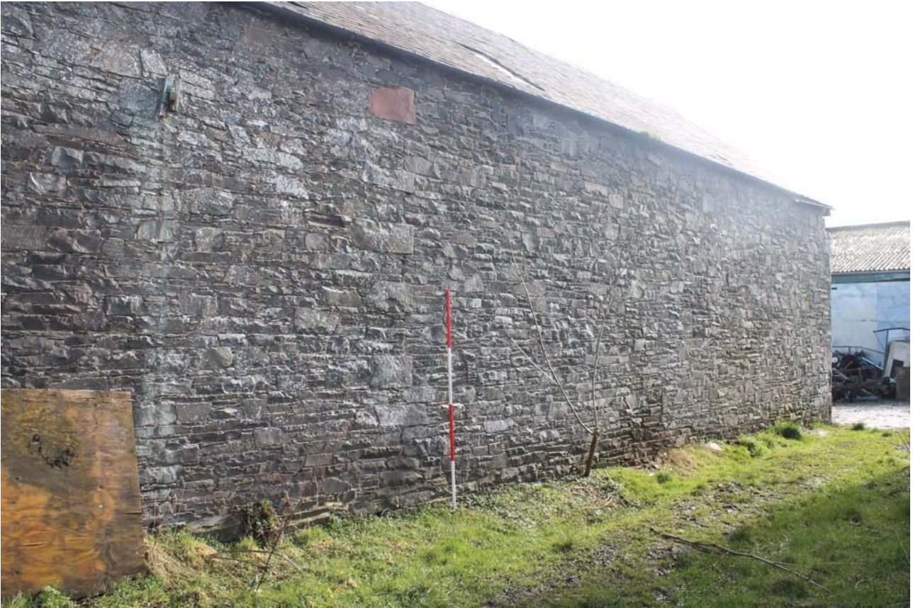
Plate 13: Barn A1, west elevation to the south side, general view from the north-west
