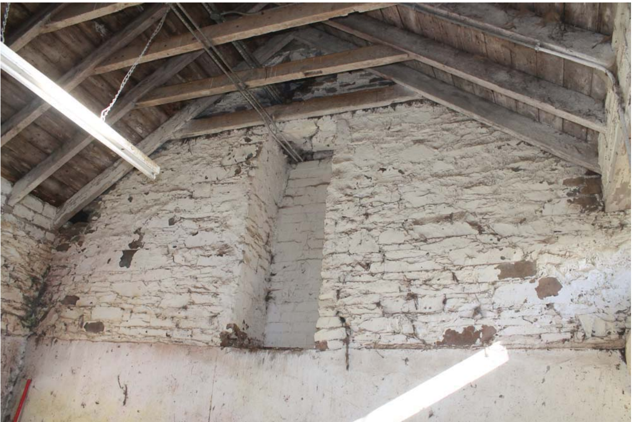
Plate 36: Barn A2/4, detail of the loading door from the hay loft in the east gable wall, from the south-west
