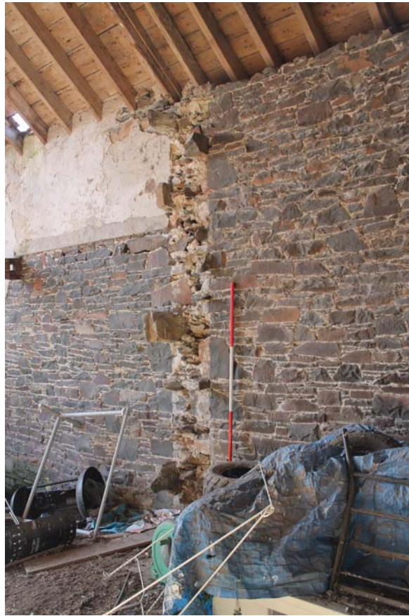
Plate 17: Barn A1/1, detail of broken-away stone partition wall to the west wall, from the north-east
