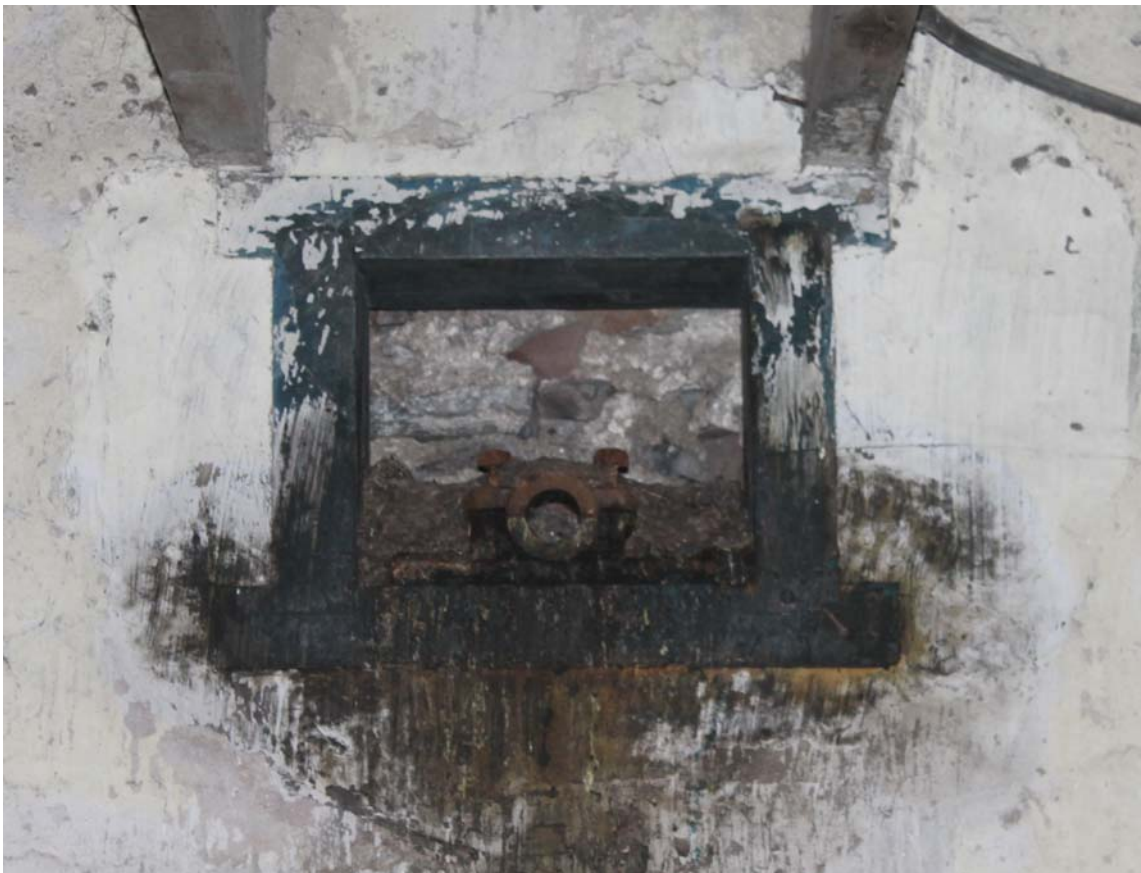
Plate 20: Barn A1/2, detail of bearing block on the east wall from the west
