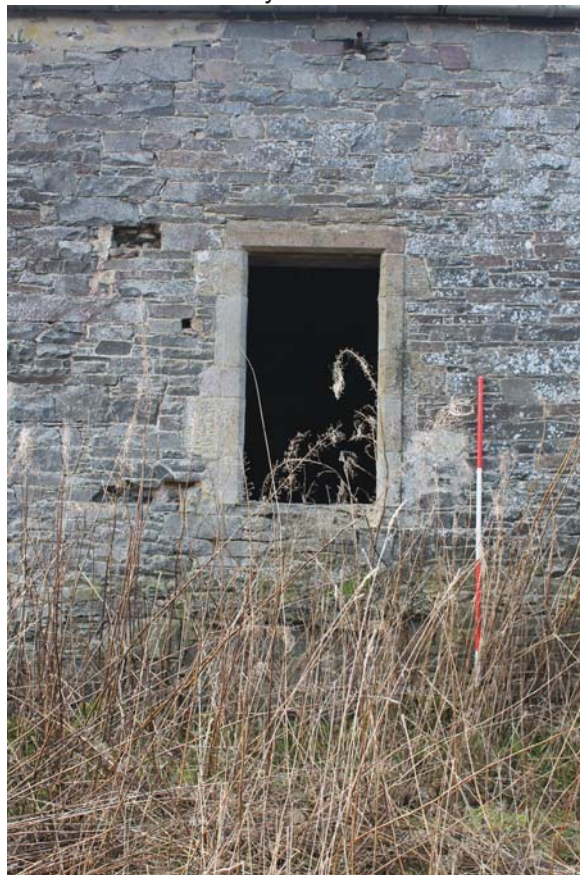
Plate 8: Barn A1, east elevation, detail of window in northernmost bay, from the east
