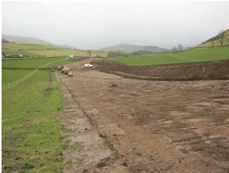
Plate 1: Post excavation view of a section of trench to the north of the TARTH Burn
