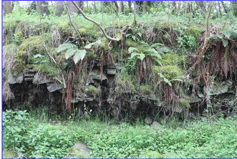
Plate 7: Detail of the remains of the mill lade wall (south side, northern end), from the north
