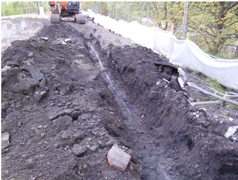
Plate 3 - General view of power cable along canal bank
