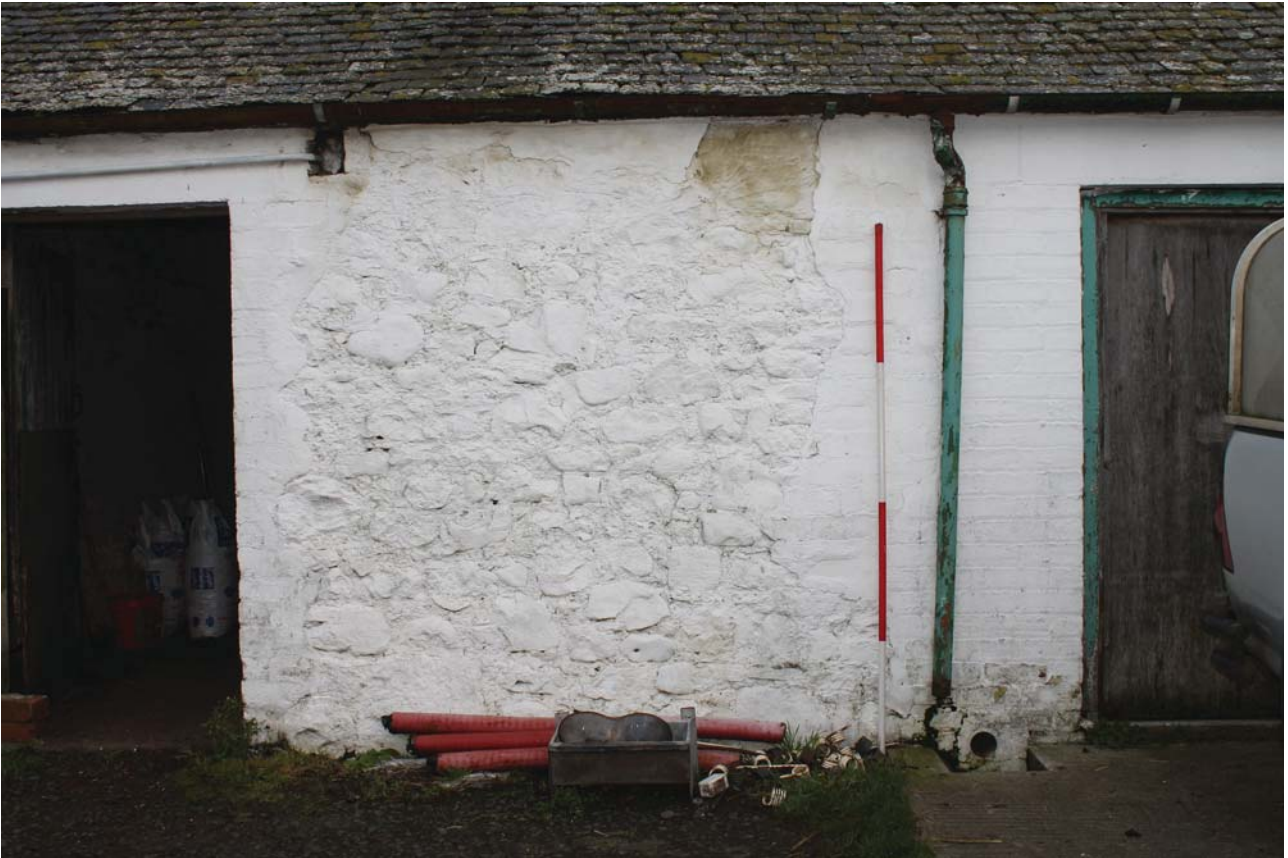
Plate 25: Laigh Corton Farm, Barn C, south-west elevation, detail of phase line from the south-west
