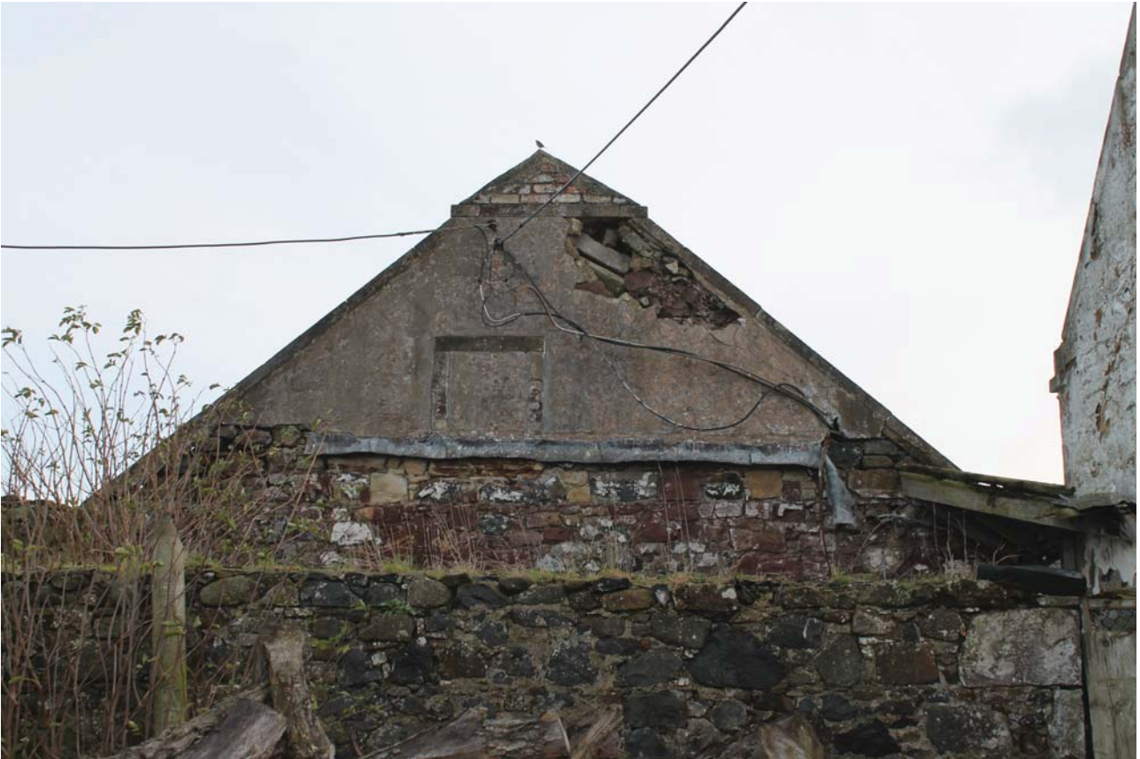
Plate 15: Laigh Corton Farm, Barn B, south-west gable, general view from the south-west
