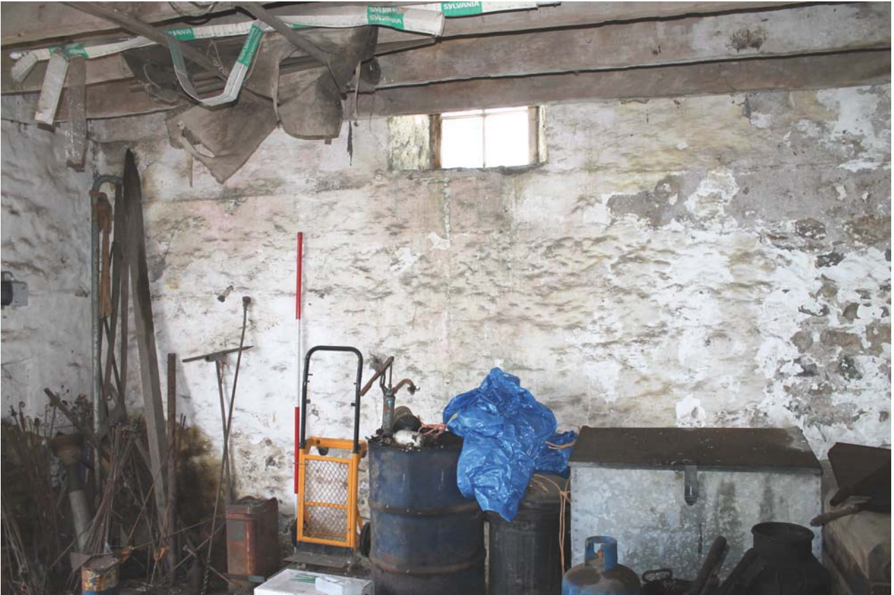
Plate 9: Laigh Corton Farm, Barn A, garage to the south-east, general view from the west
