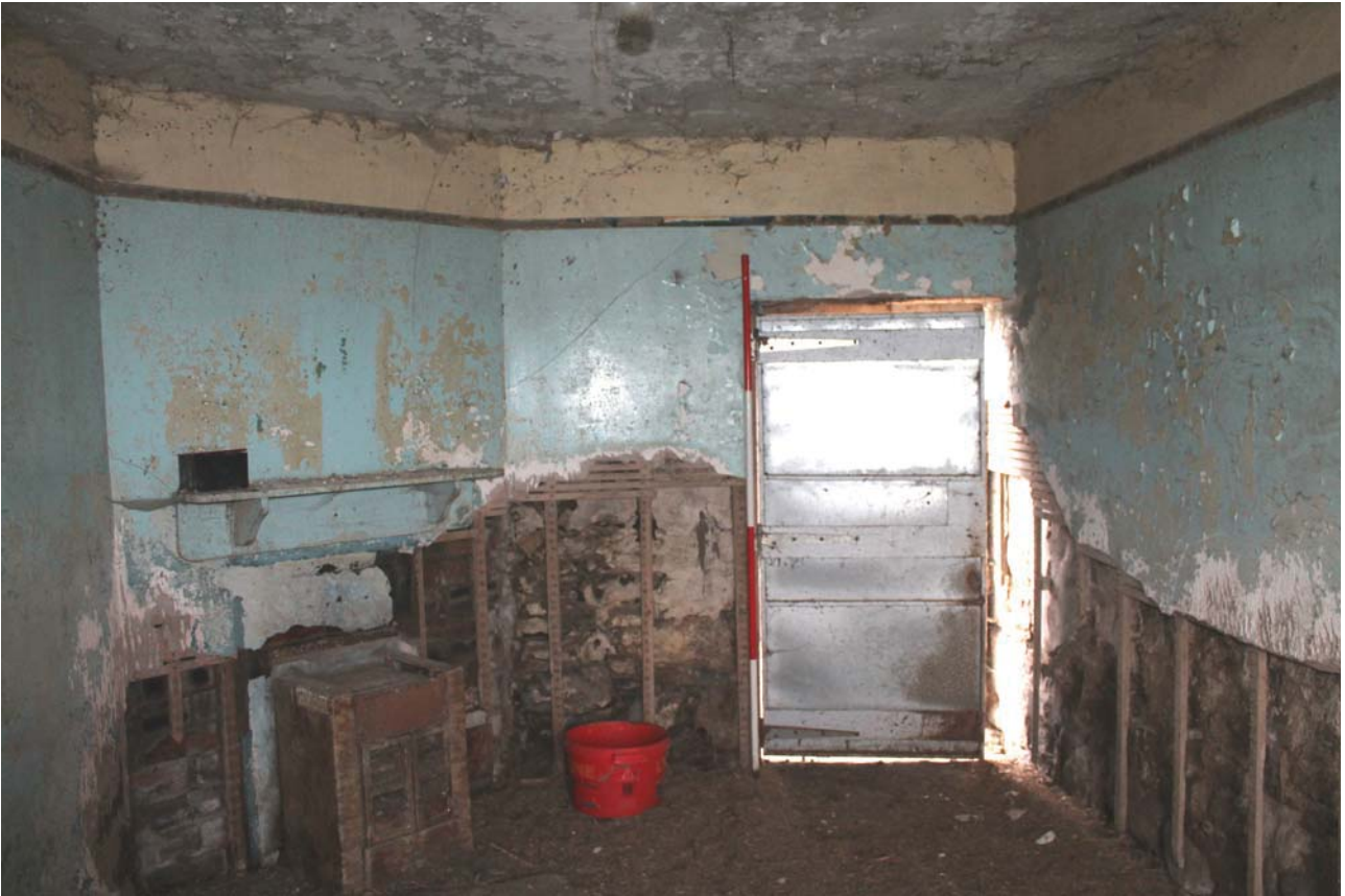
Plate 33: Laigh Corton Farm, Barn C, detail of central room showing blocked corner fireplace from the north-east
