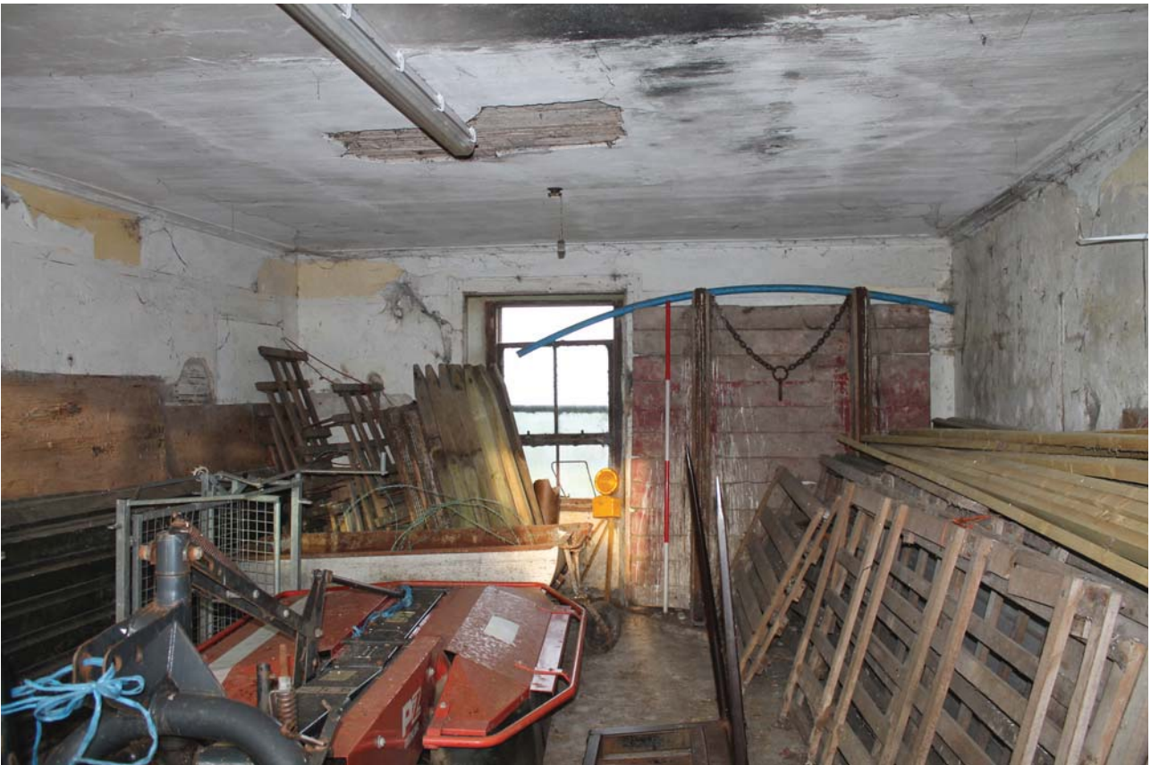
Plate 22: Laigh Corton Farm, Barn B, general view of the ground floor south-westernmost room from the south-east
