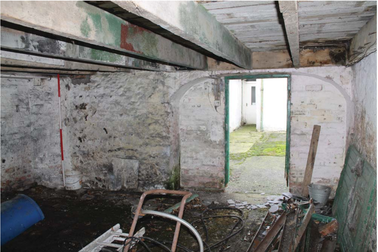
Plate 55: High Corton Farm, Barn C, detail of the cart entrance on the north-west wall of the south-west barn from the south-east
