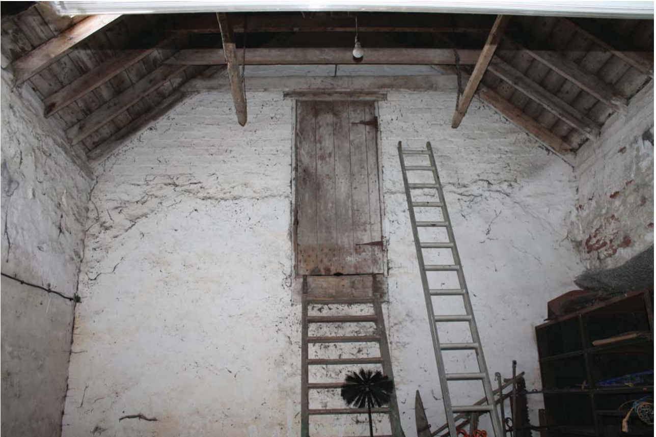
Plate 11: Laigh Corton Farm, Barn A, store to the north-west, general view looking at hay loft doorway from the north-west
