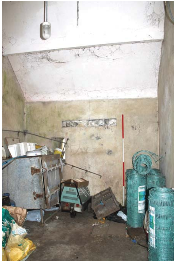
Plate 30: Laigh Corton Farm, Barn C, detail of north-westernmost room from the south-west
