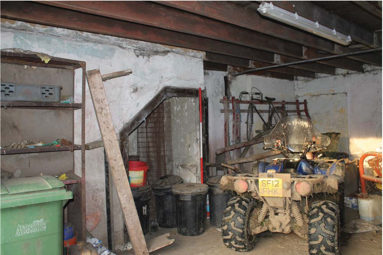
Plate 19: Laigh Corton Farm, Barn B, detail of the ground floor north-westernmost room, showing understair cupboard, from the east
