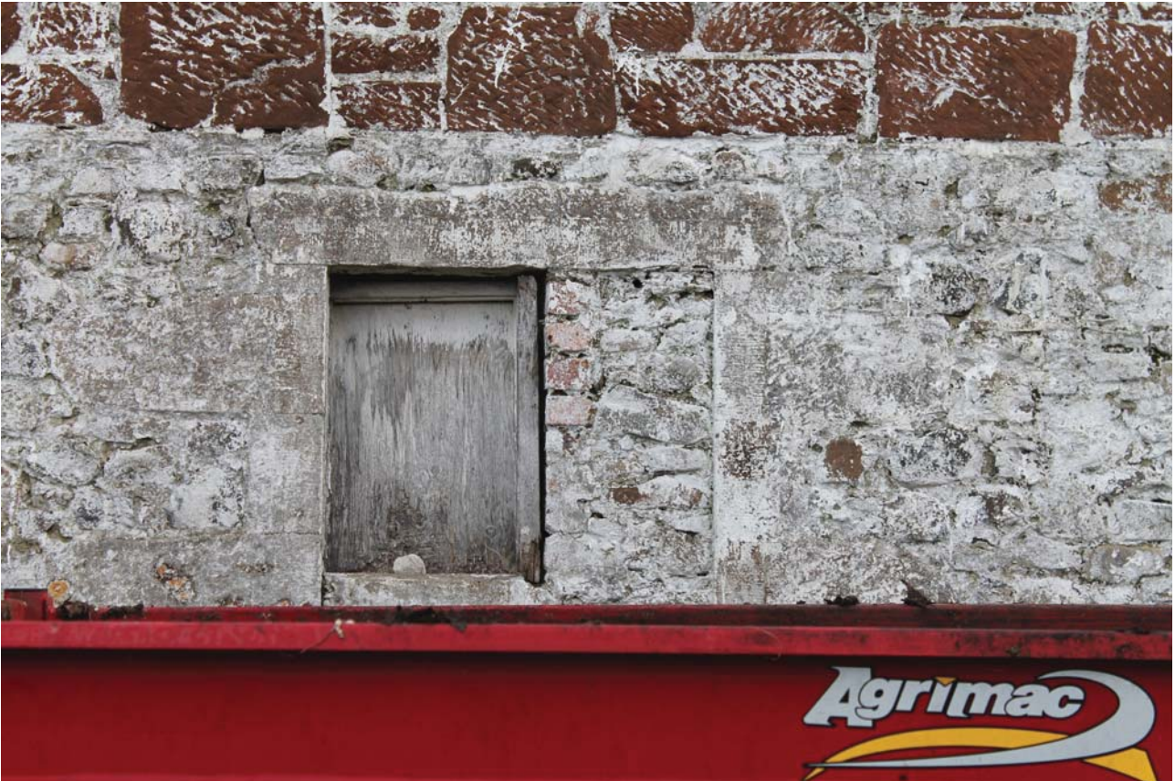
Plate 5: Laigh Corton Farm, Barn A, detail of window inserted into blocked doorway from the south-west
