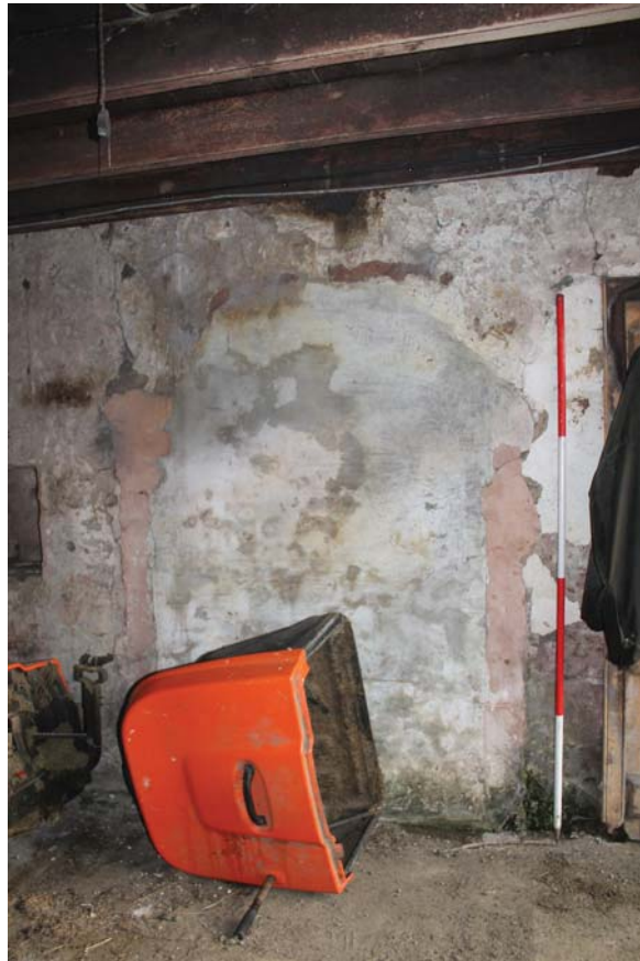
Plate 21: Laigh Corton Farm, Barn B, detail of the ground floor north-westernmost room, showing blocked doorway, from the SWW
