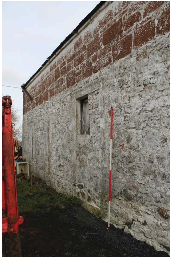
Plate 4: Laigh Corton Farm, Barn A, south-west elevation, detail of blocked doorway from the south
