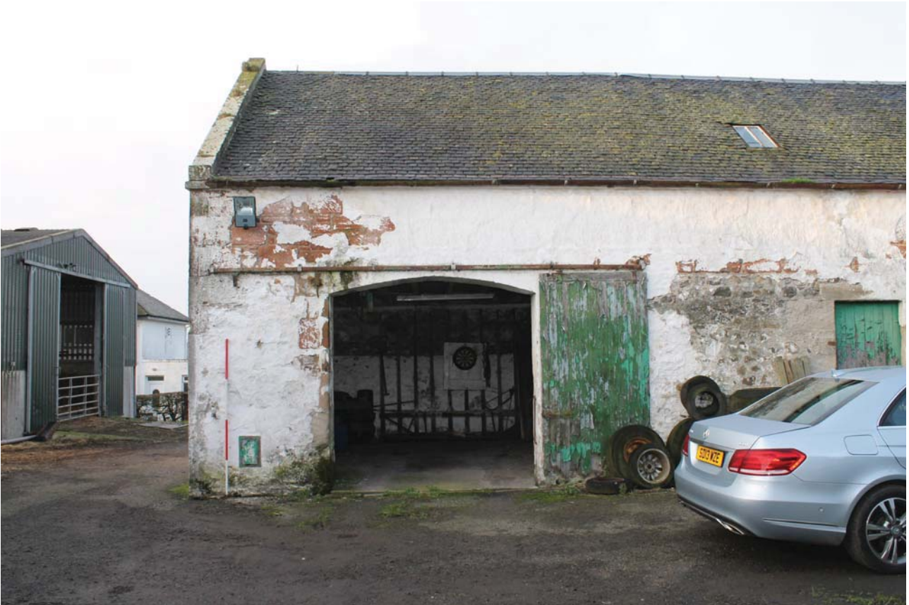
Plate 3: Laigh Corton Farm, Barn A, north-east elevation, detail of cart entrance from the north-east
