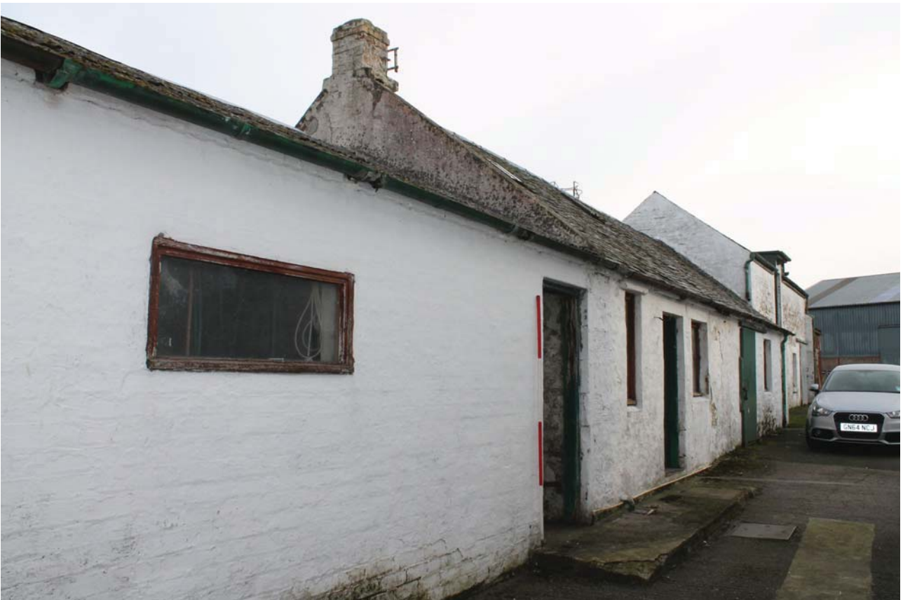
Plate 58: High Corton Farm, Barn D, south-west elevation, general view of the north-west end from the west
