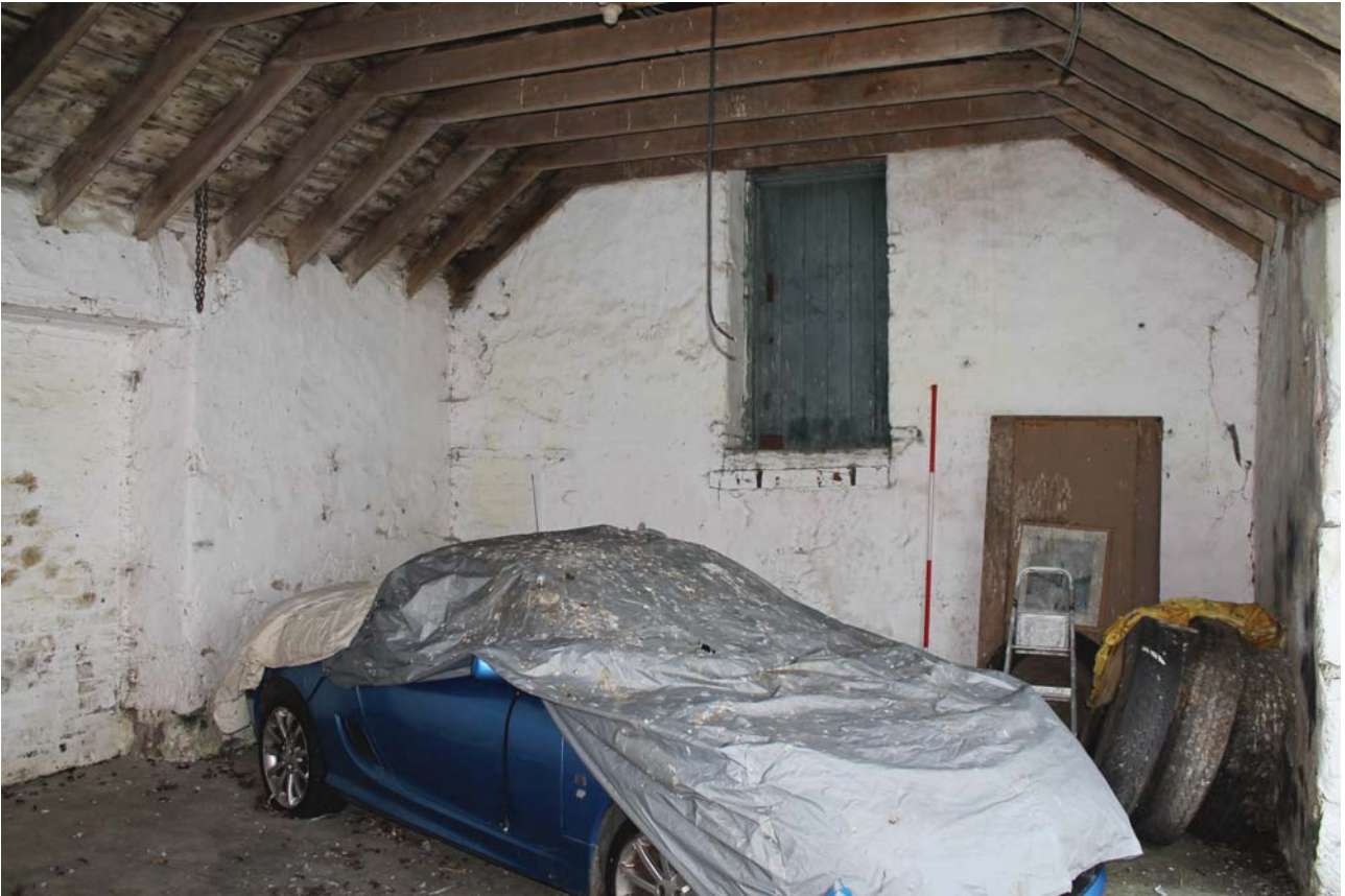
Plate 53: High Corton Farm, Barn C, detail of hay loft door in the south-west wall of the north-east garage, from the north-east
