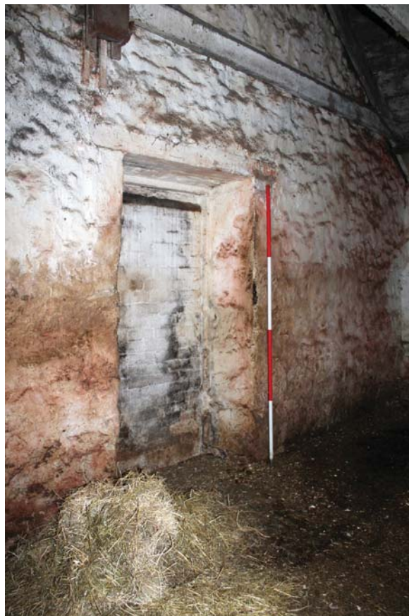
Plate 48: High Corton Farm, Barn B, detail of blocked doorway in the north-west wall from the south
