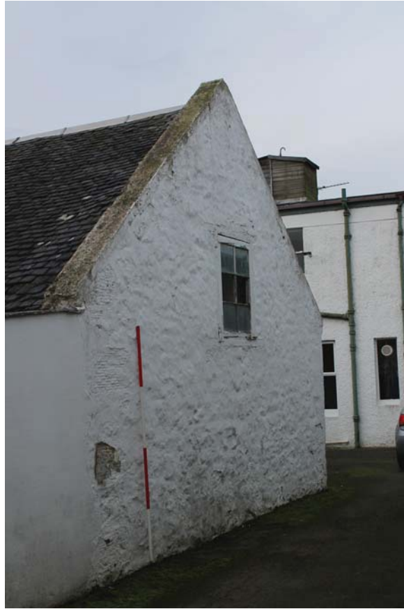
Plate 51: High Corton Farm, Barn C, general view of the north-east gable from the east
