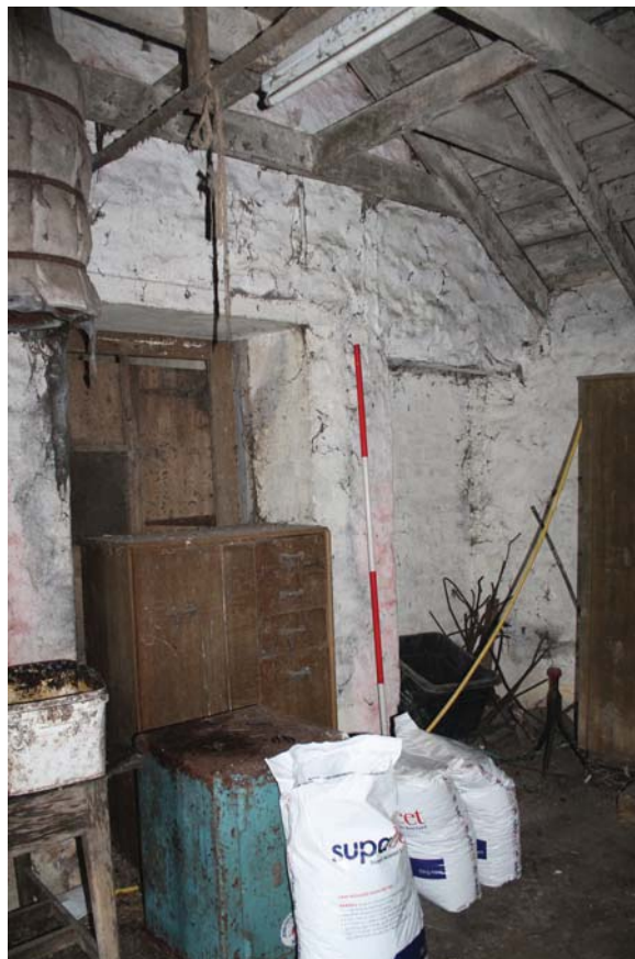
Plate 46: High Corton Farm, Barn B, detail of blocked openings on the north-east wall from the west
