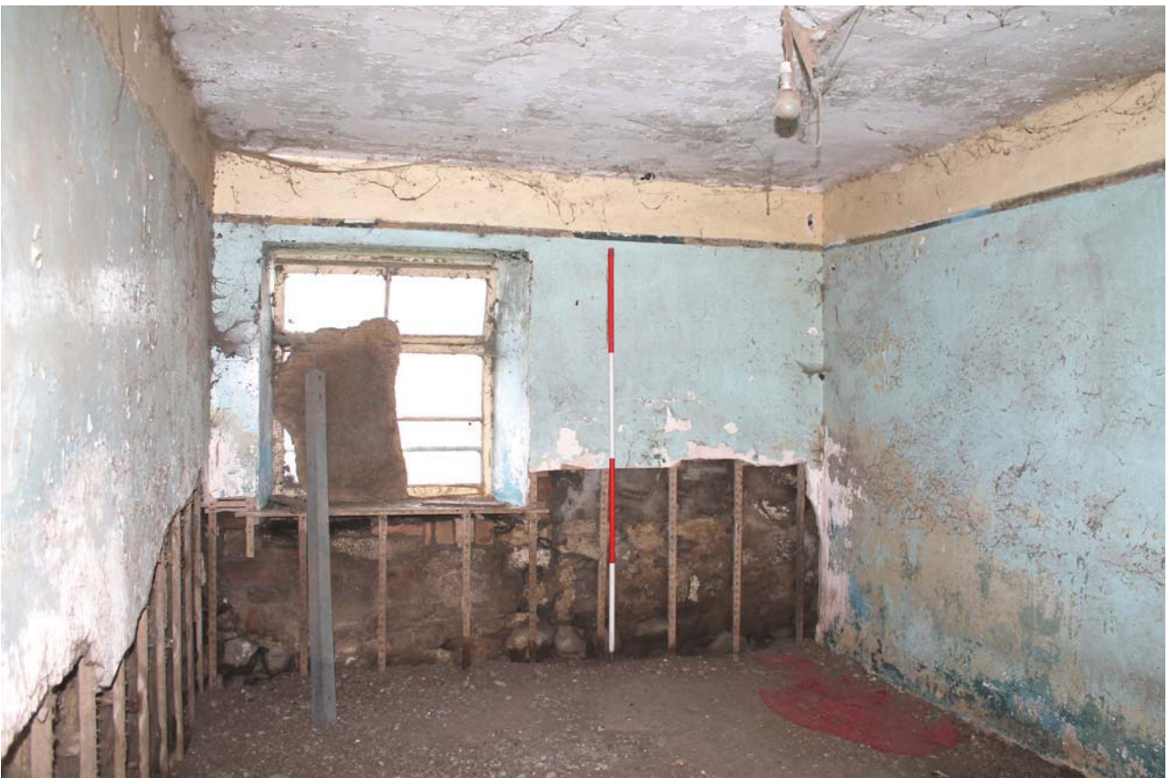
Plate 32: Laigh Corton Farm, Barn C, detail of central room from the south-west
