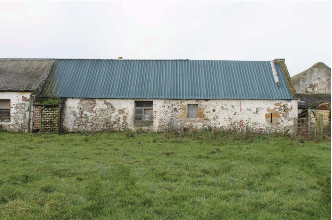
Plate 27: Laigh Corton Farm, Barn C, north-east elevation, general view from the north-east
