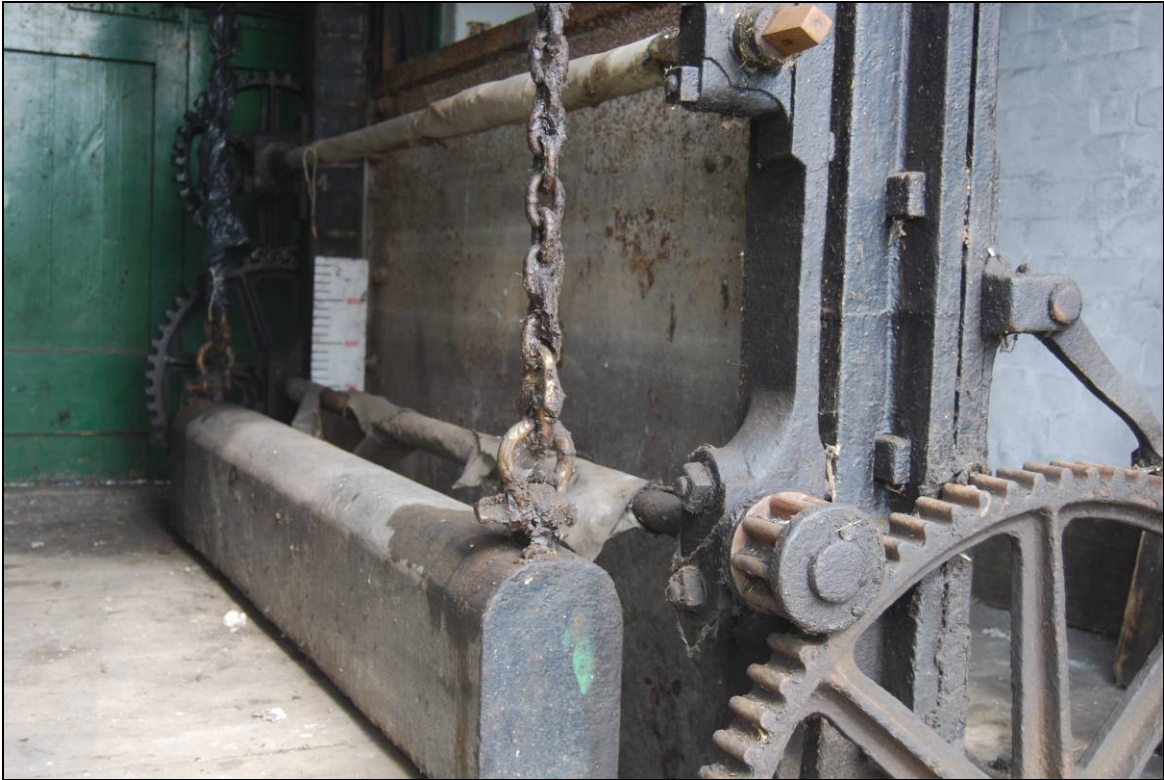
Plate 14: Sluice Mechanism Including Counter-weight
