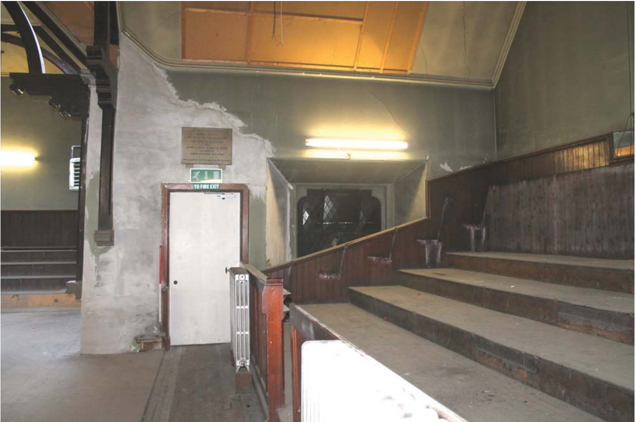
Plate 77: Room 1/1, general view of the south-west wall of the north-west transept from the north-east
