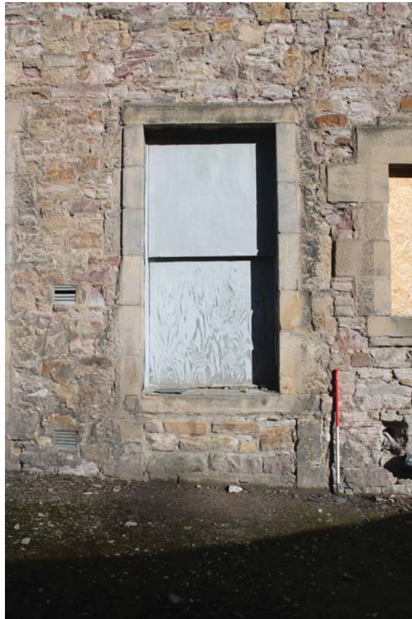
Plate 23: South-west elevation, detail of the central window, showing blocking beneath, from the south-west
