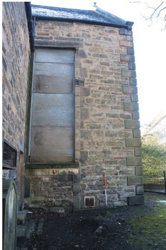
Plate 16: North-west transept, north-east elevation, detail of the large window and blocking beneath, from the north-east
