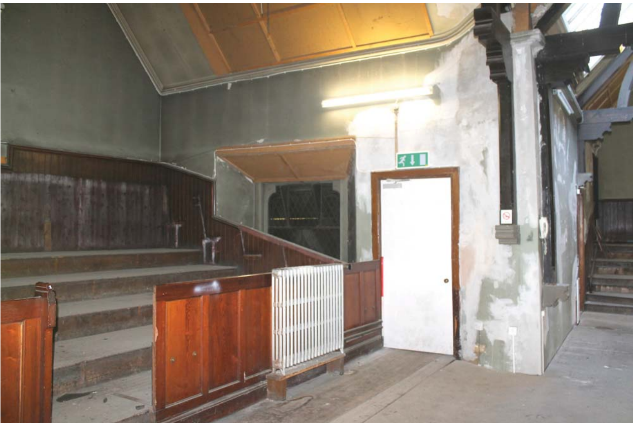
Plate 76: Room 1/1, general view of north-east wall of the north-west transept from the south
