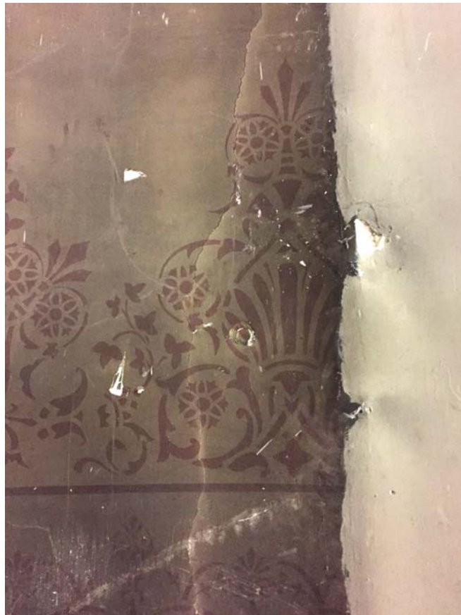
Plate 90: Room 0/1, detail of decorative plasterwork in the north-west wall after the removal of the organ, from the south
