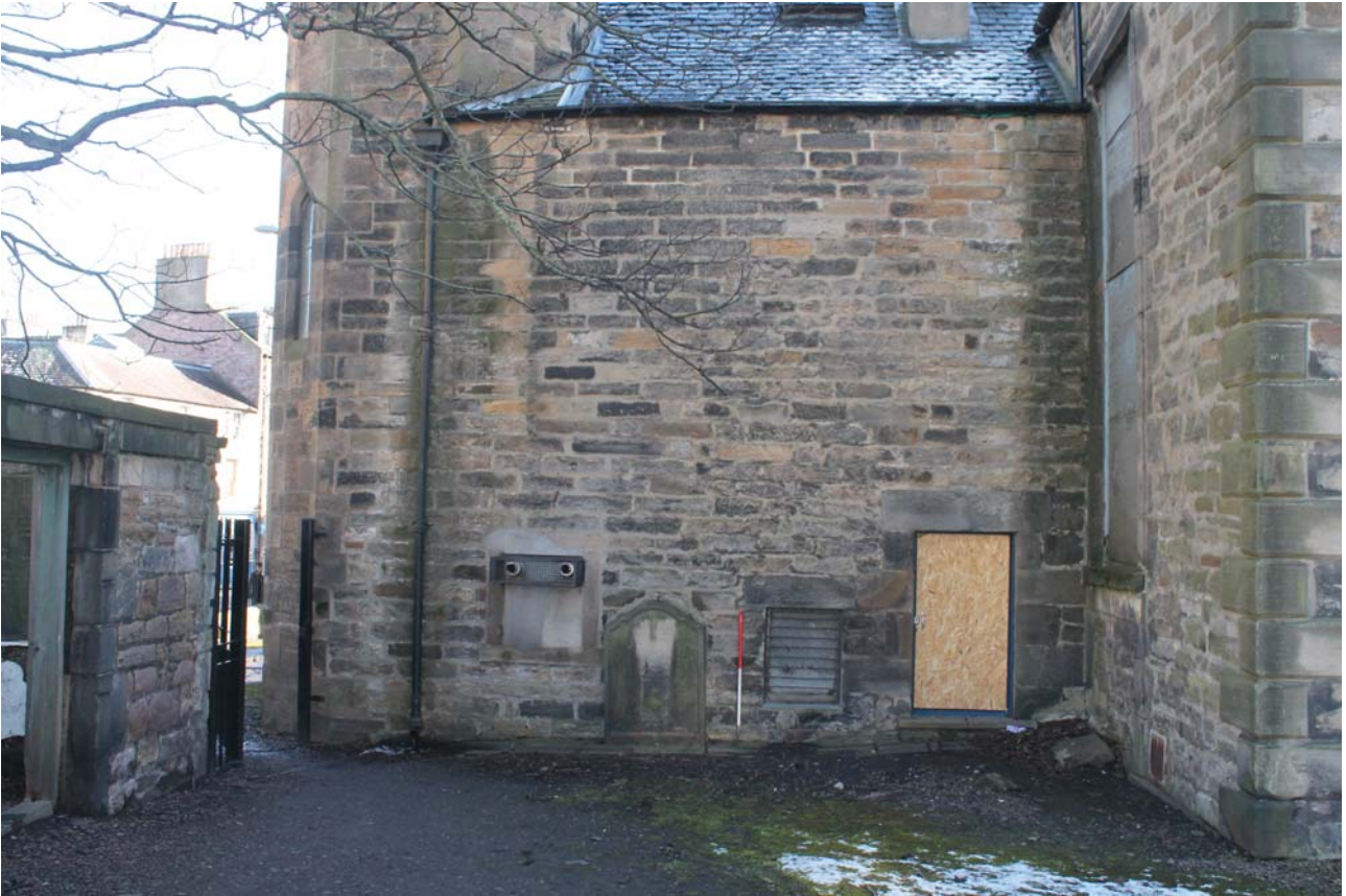
Plate 17: North-west elevation, general view of the openings to the Boiler House on the north-east side, from the north-west
