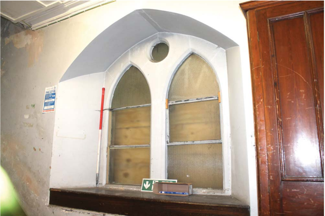
Plate 53: Room 0/2, detail of window in the north-east wall to the north-west side of the porch, from the west
