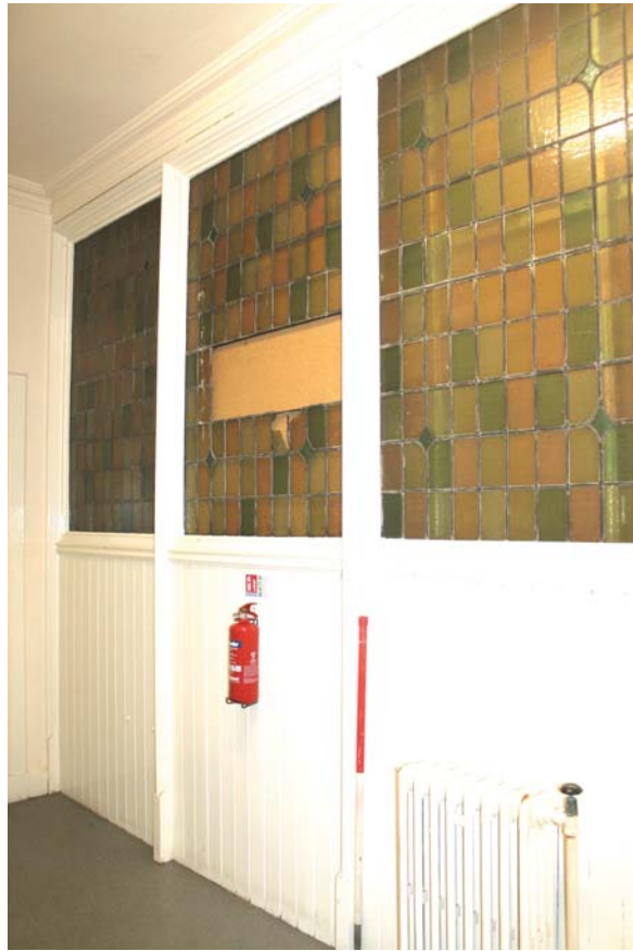
Plate 61: Room 0/5, general view of partition glazing in the north-east wall from the south
