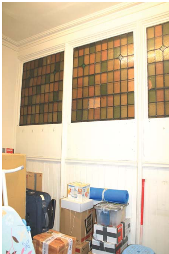
Plate 54: Room 0/3, general view of south-west wall and glazed panelling from the north
