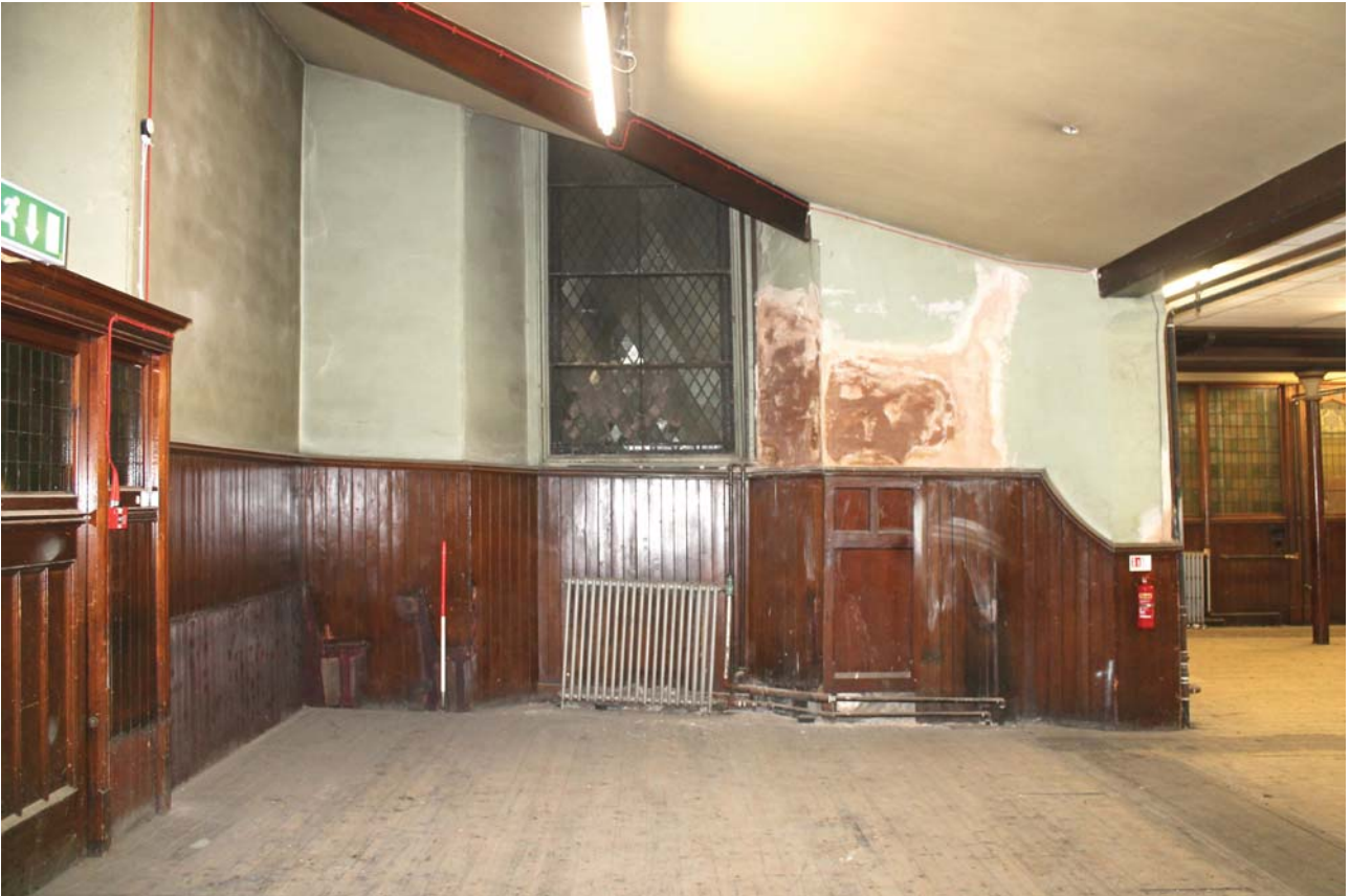
Plate 47: Room 0/1, detail of the window on the north-east wall of the north-west transept, from the south-west
