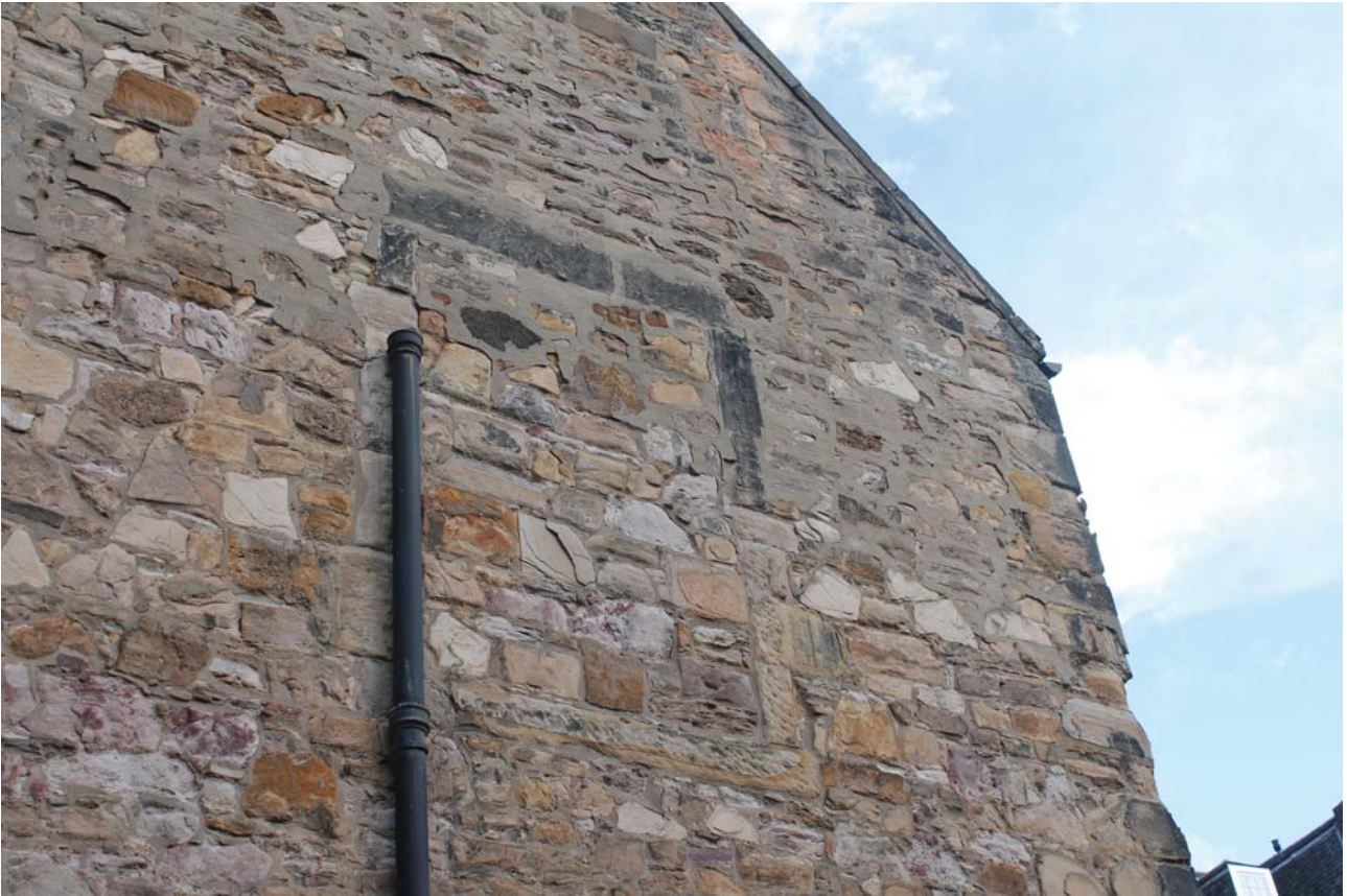
Plate 21: South-west elevation, detail of the blocked first floor window on the south-east side, from the west
