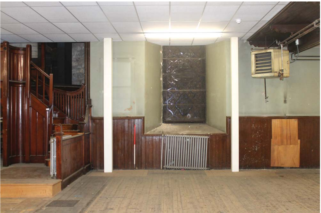
Plate 44: Room 0/1, detail of the window on the south-west side of the south-east wall from the north-west
