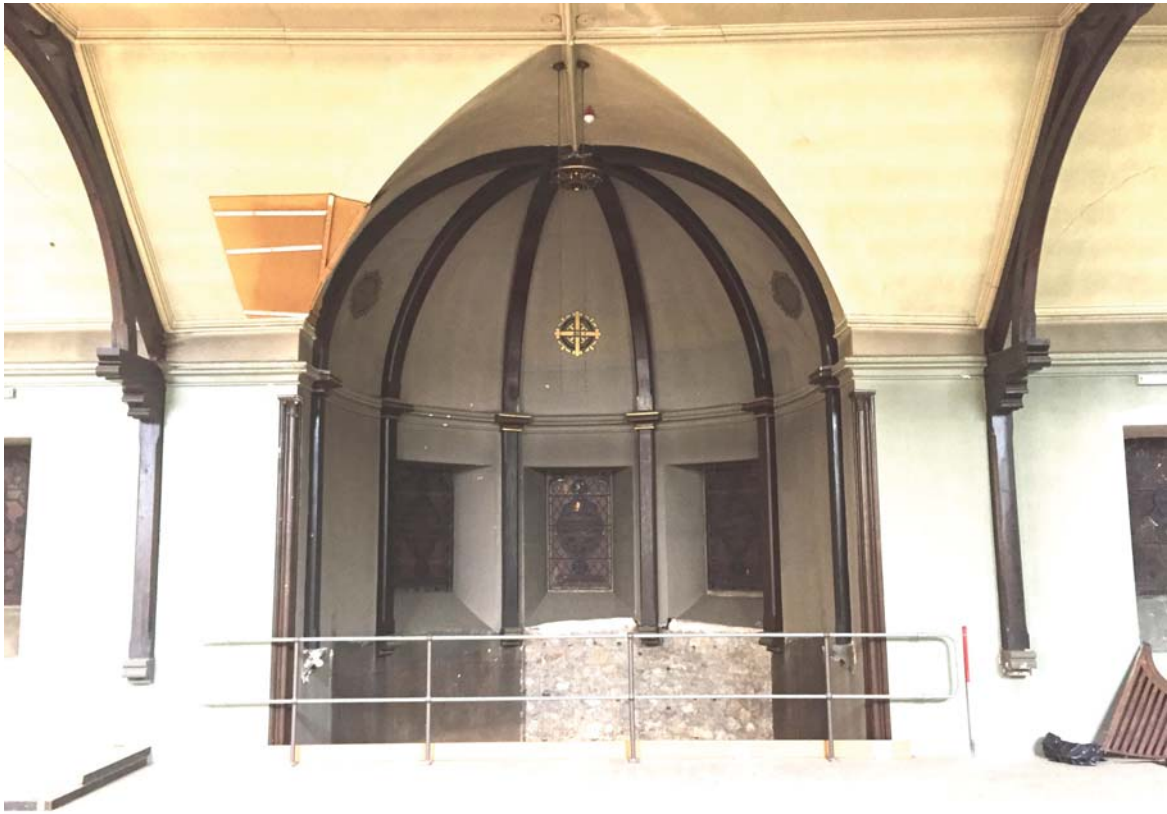
Plate 91: Room 1/1, general view of the north-west wall after the removal of the organ, from the south-east
