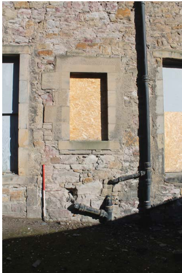
Plate 22: South-west elevation, detail of the inserted toilet window on the south-east side, from the south-west
