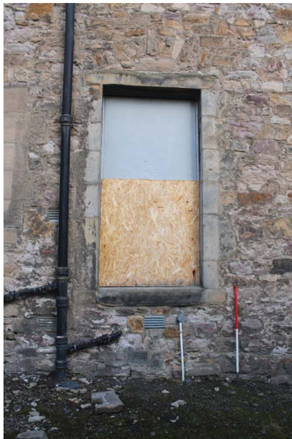
Plate 20: South-west elevation, detail of the window on the south-east side from the south-west
