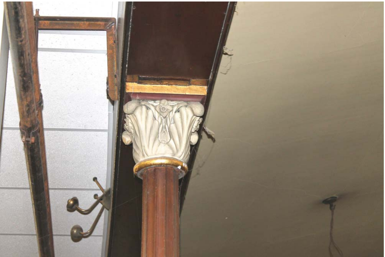
Plate 33: Room 0/1, detail of column head in front of the north-west transept from the east
