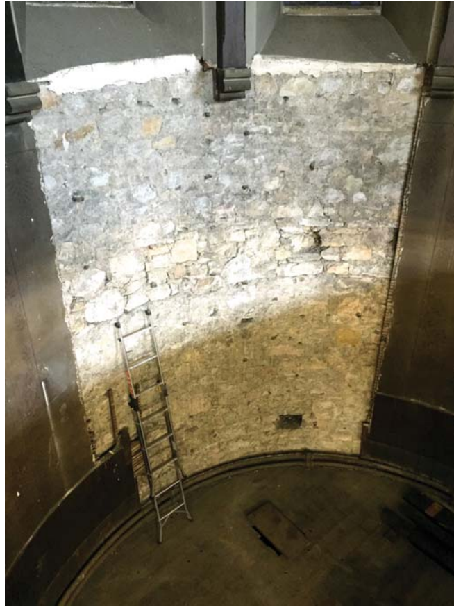
Plate 87: Room 0/1, general view of the exposed stone rubble wall looking down from Room 1/1 after the removal of the organ, from the south
