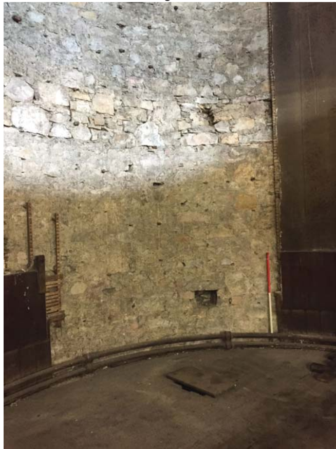
Plate 88: Room 0/1, general view of the exposed stone rubble wall after the removal of the organ, from the south
