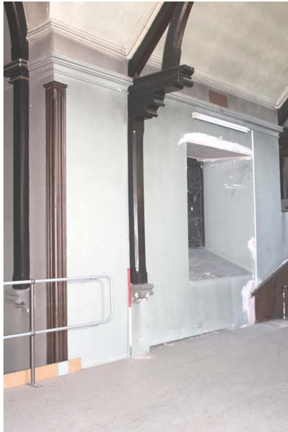
Plate 79: Room 1/1, detail of moulded timber rafter on the south-east wall from the north
