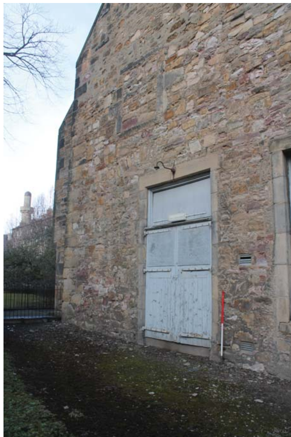
Plate 24: South-west elevation, detail of the main doorway to the north-west side showing the original blocked entrance from the west
