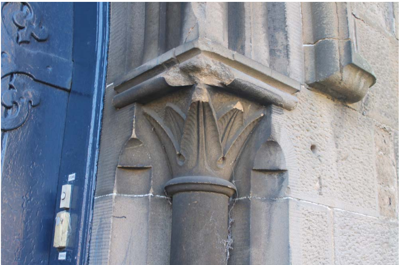
Plate 4: North-east elevation, detail of column head on the north-west side, from the east
