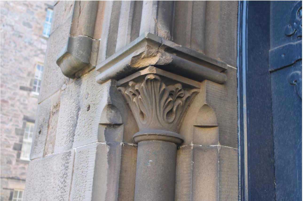
Plate 5: North-east elevation, detail of column head on the south-east side, from the north
