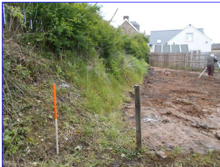
Plate 2: General view of difference in ground level from plots to the north
