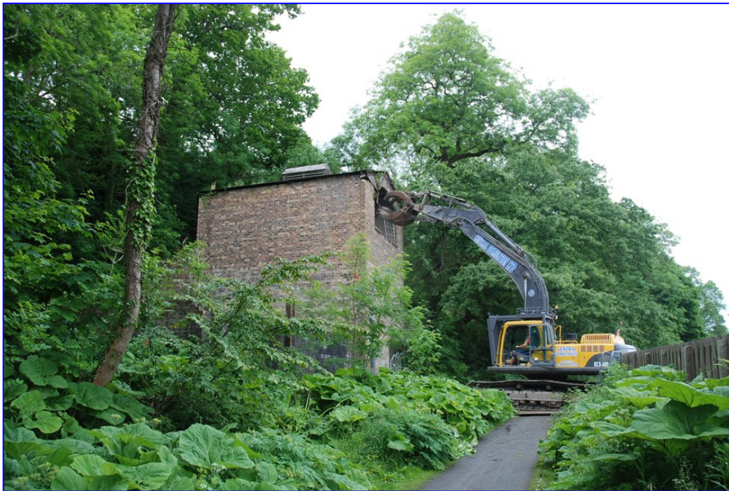
Plate 7: General view of the building just as it was being demolished, from the north-east
