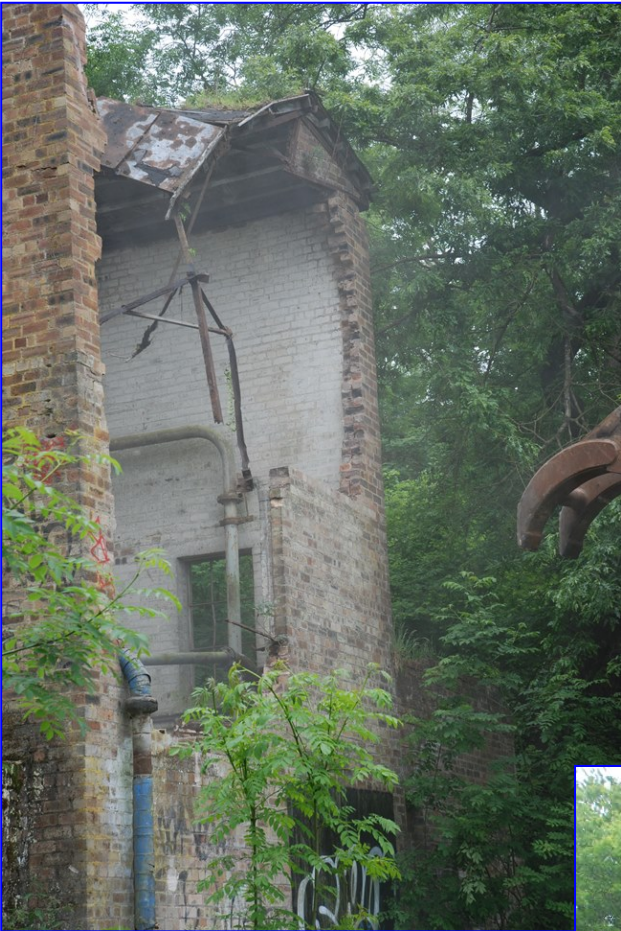
Plate 8: General view of the building after the demolition of the north wall exposing the white-washed brick interior, from the north-east
