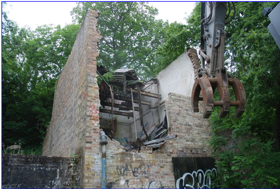
Plate 10: General view of the demolition showing the steel beams supporting the roof from the NNE
