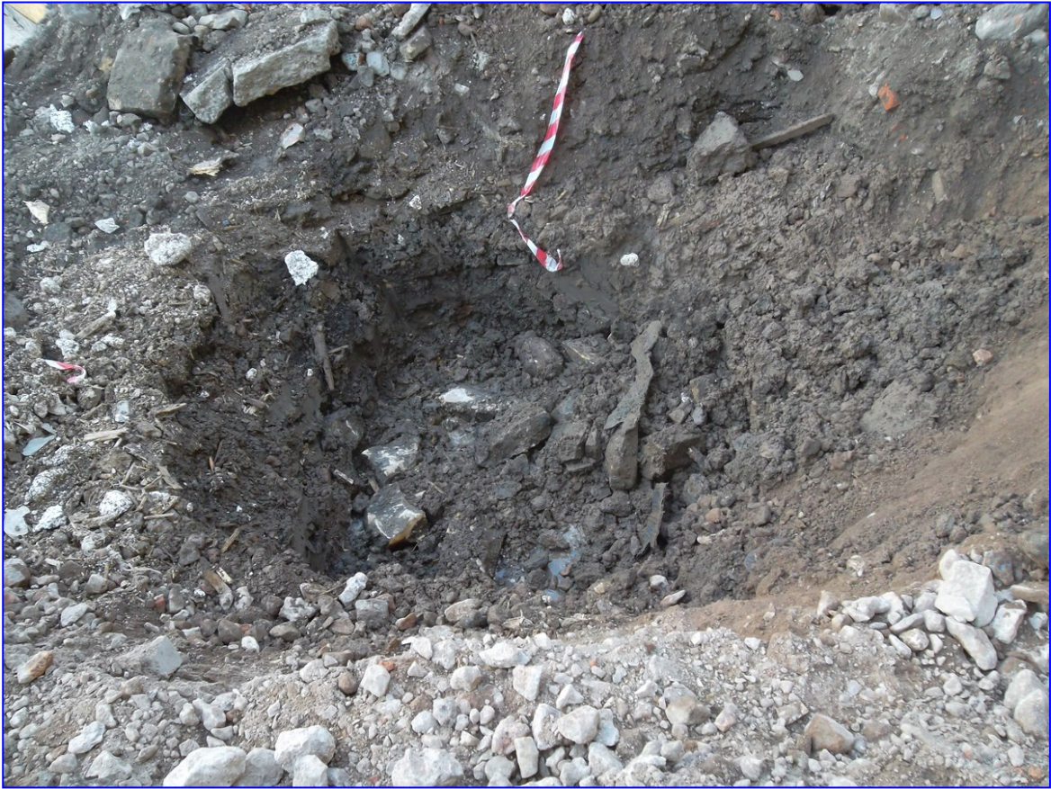
Plate 17: General view after removal of the top 1m of the well which was then filled in and later capped with concrete
