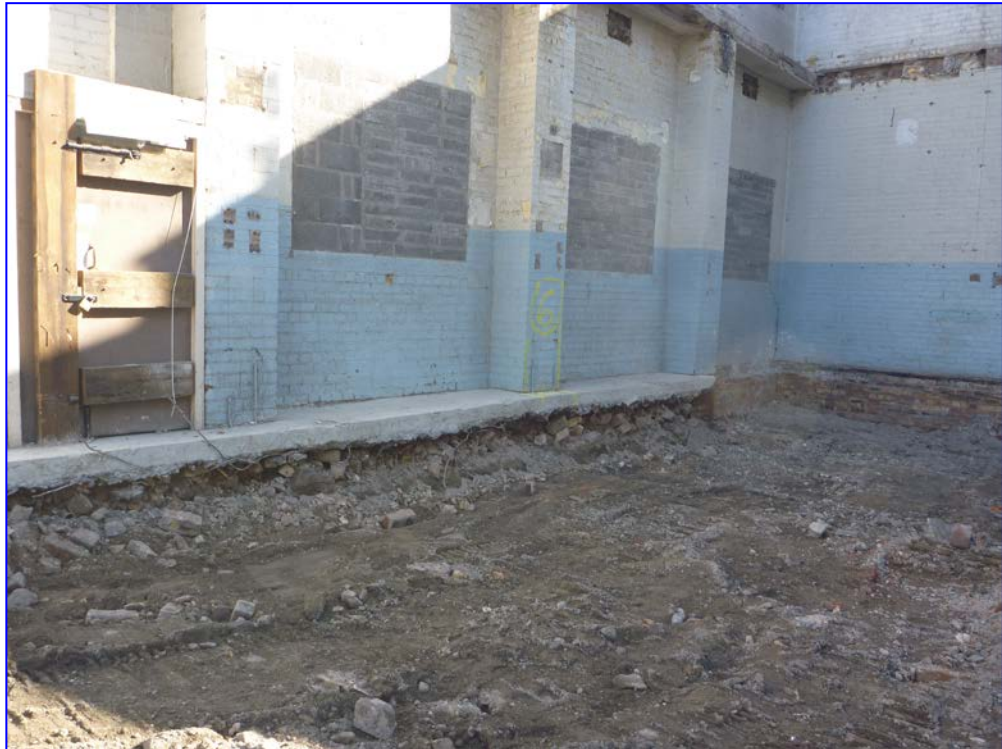
Plate 1: General view of the excavation of the concrete floor slab from the south showing made ground rubble (000) over the site prior to the excavation of the test pits
